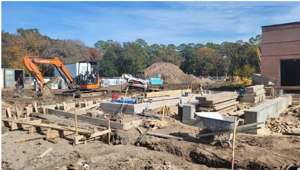
Generator and Chiller Pads at Service Yard
