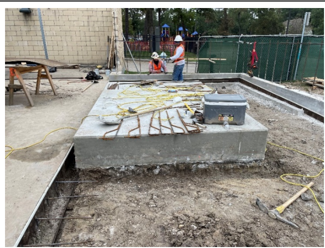
Item #02: Chiller concrete pad at the mechanical yard.
