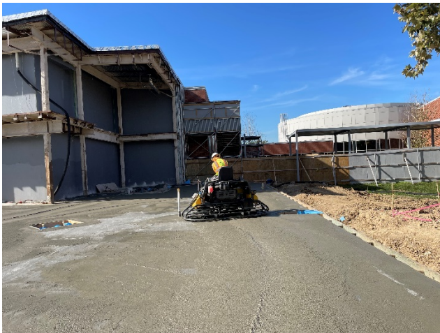
Item #03: Power trowels were used to bring the concrete to a smooth finish.
