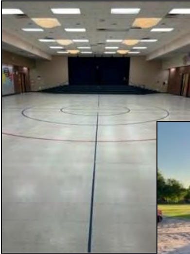
Polished Concrete Floors
