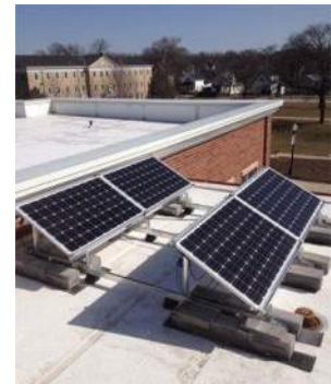
Photovoltaic panels at Elgin Academy
