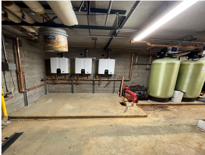
New Water Heaters
