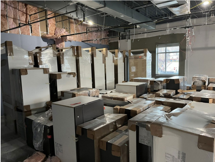
Cabinets Delivered On-Site
