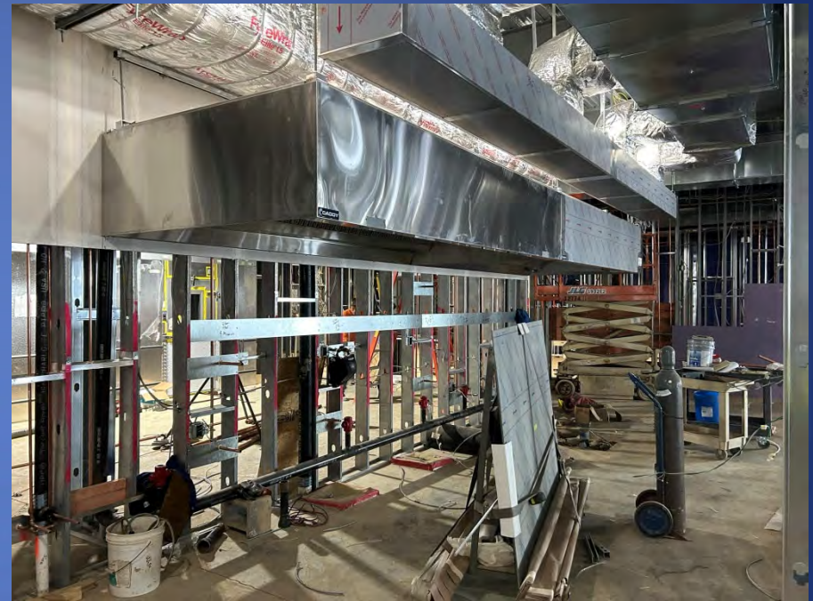
Duct Work for Oven and Stovetop
