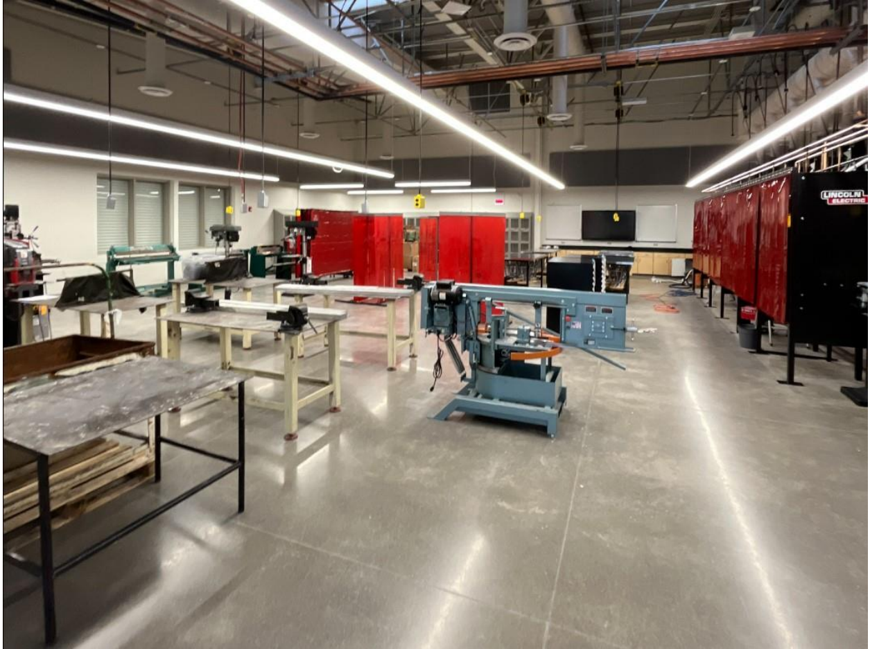
Metal shop with equipment in its final locations
