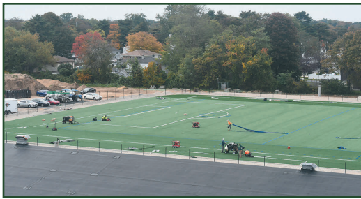
One of the larger capital improvement projects was the creation of a brand-new turf soccer field next to the Anthony F. Felicio Administration Building. Upon completion, the complex will feature lights and a community track in addition to a state-of-the-art surface for varsity soccer matches.
