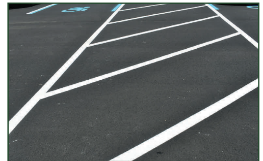
Progress in the parking lot at Loretta Park Elementary School over the summer.
