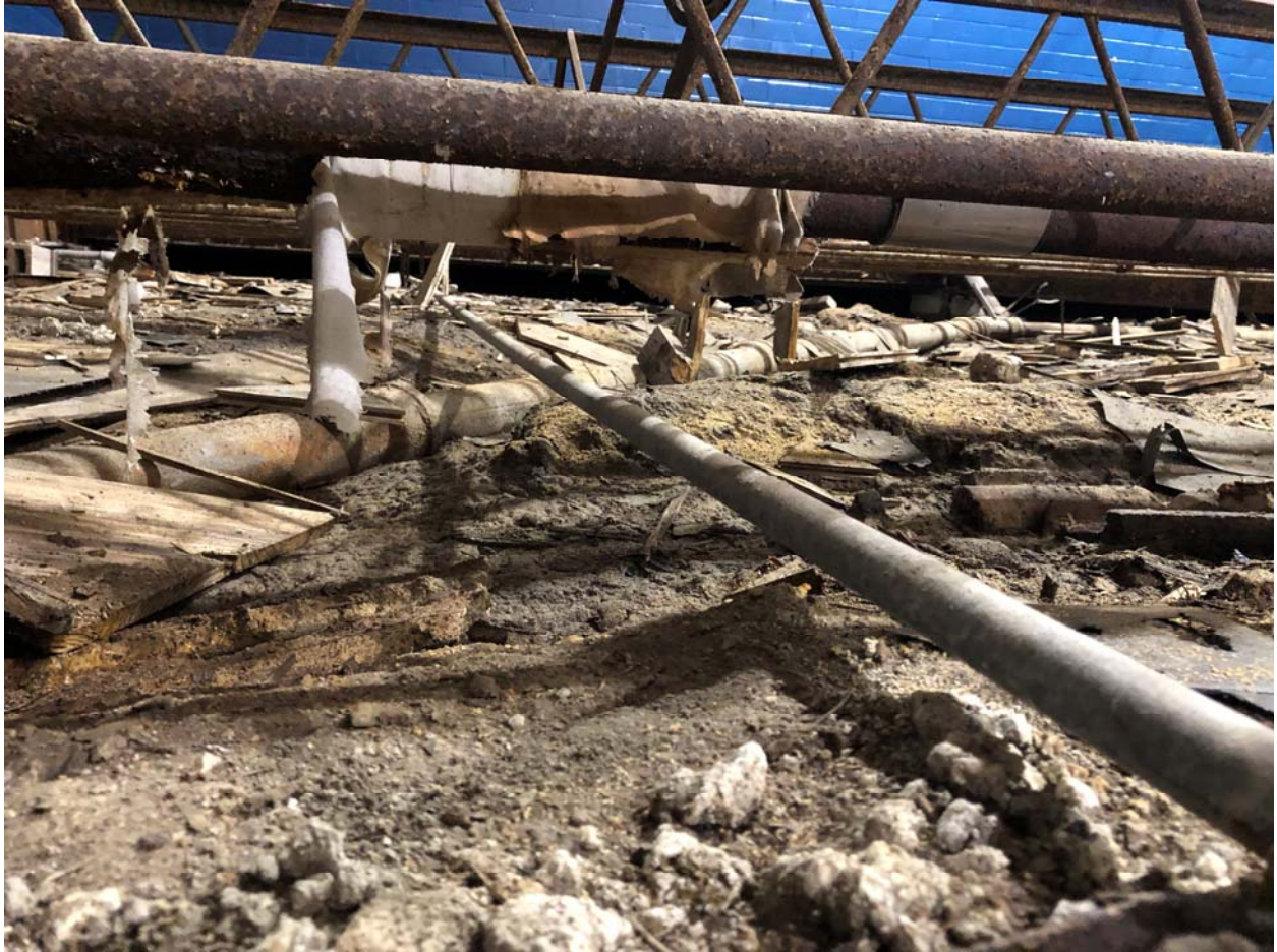
Crawlspace TSI & Debris
