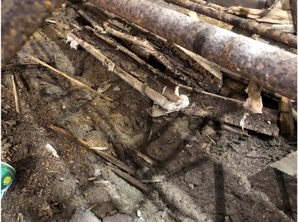
Crawlspace TSI & Debris
