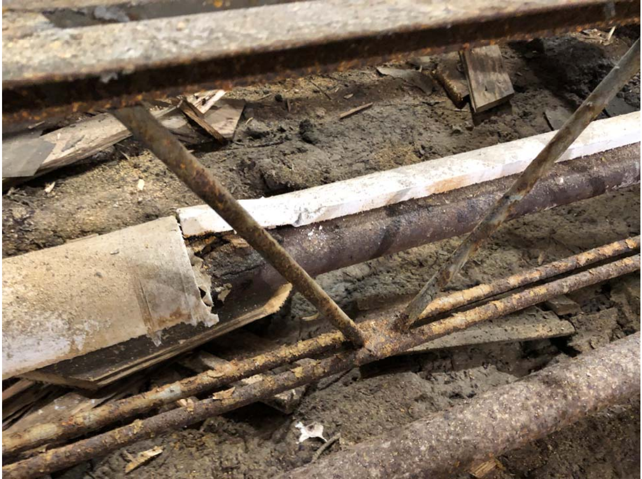
Crawlspace TSI & Debris
