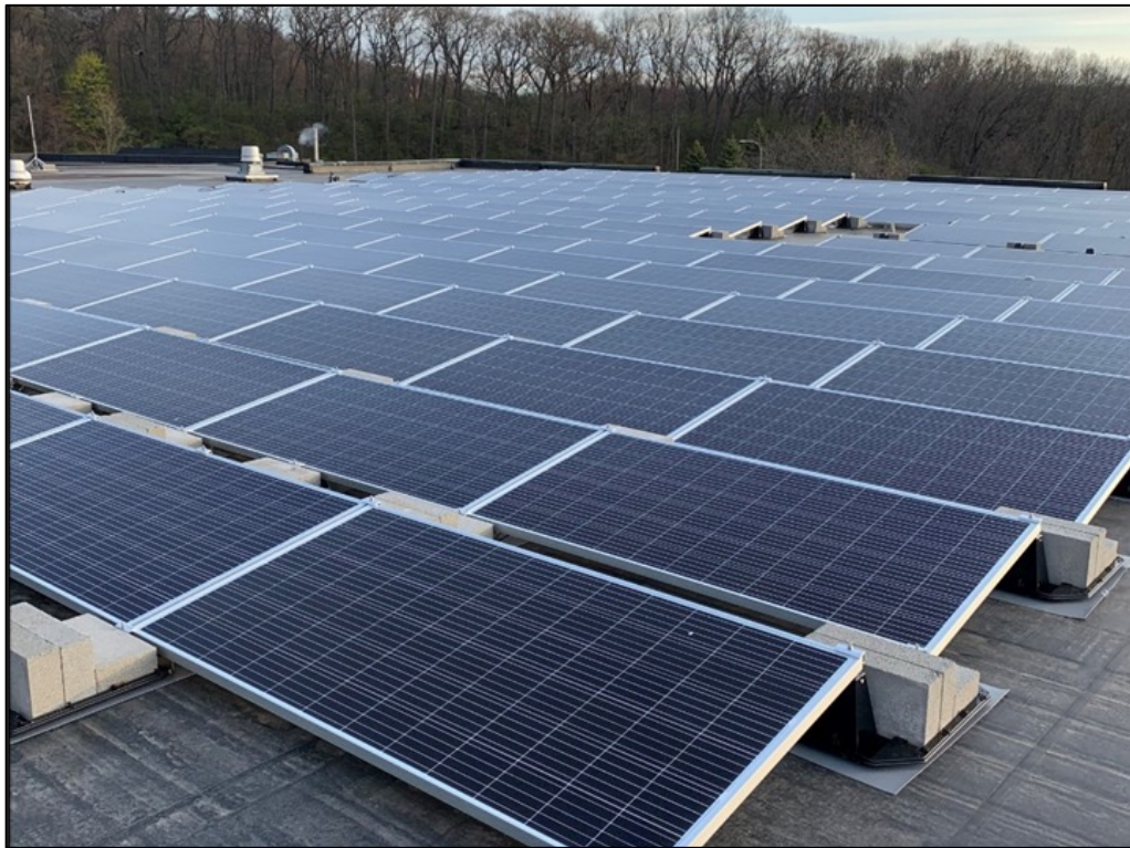
- Huron High School Solar
