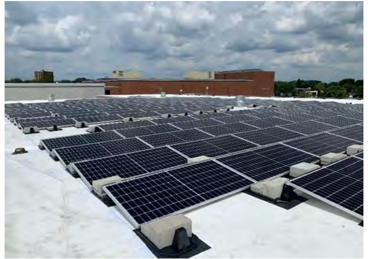
Pioneer High School – Solar Array
