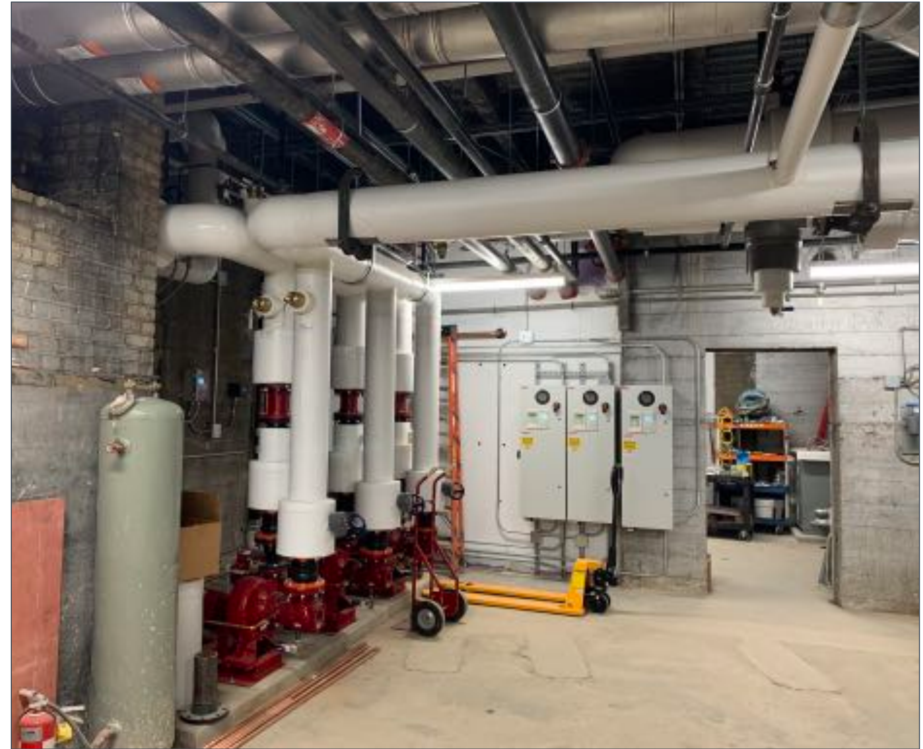
- New Pumps and Piping
