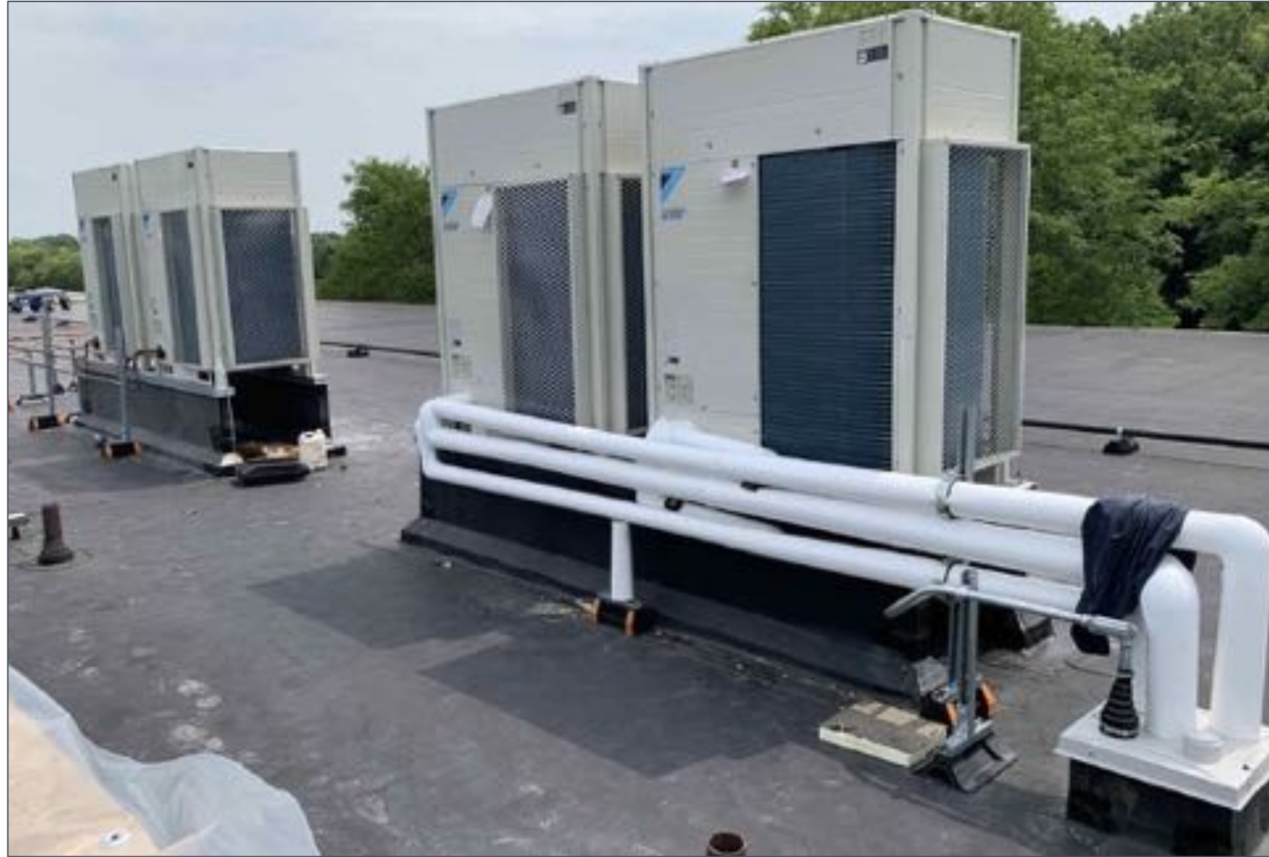
- New Condensing Units
