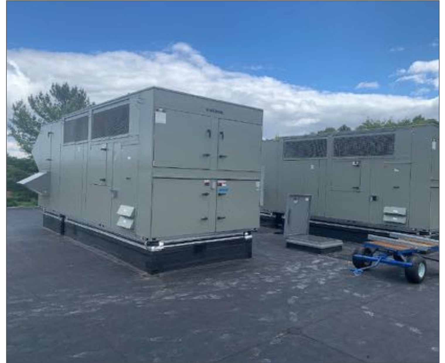
- New Ventilation Equipment
