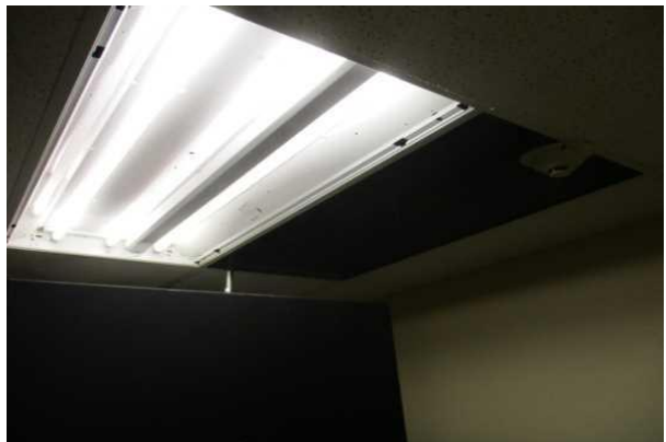
#30: MISSING CEILING TILES
