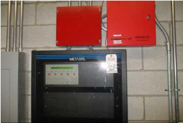
#49: FIRE ALARM PANEL
