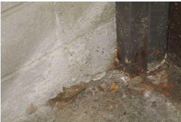
#17: EXTERIOR DOOR FRAME DAMAGE
