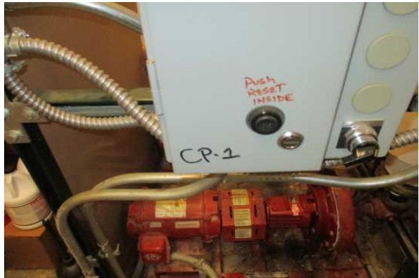
#40: DISTRIBUTION PUMP, HEATING WATER
