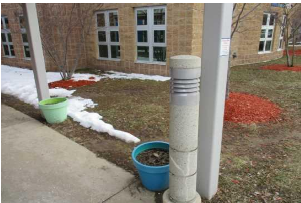
#65: WALKWAY BOLLARD LIGHT
