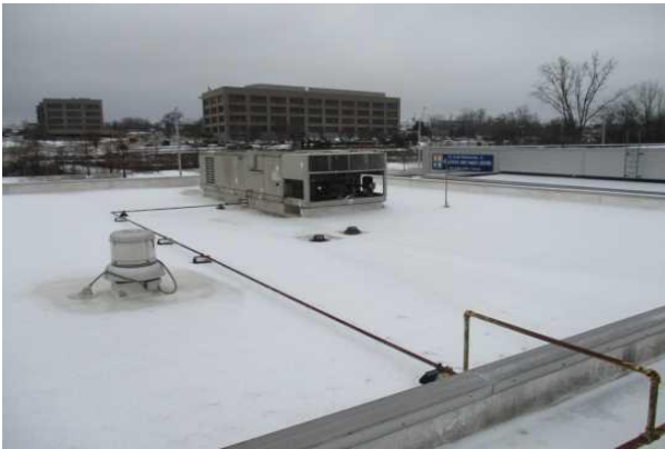
#15: RTU AND GAS PIPING ON ROOF
