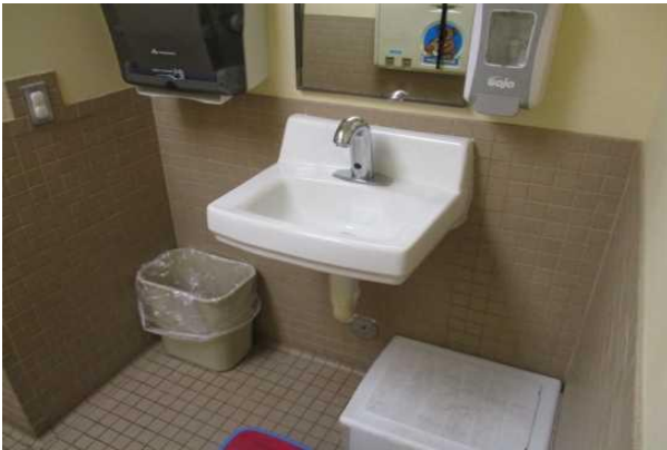
#33: SINK WITH WRAPPED PIPE
