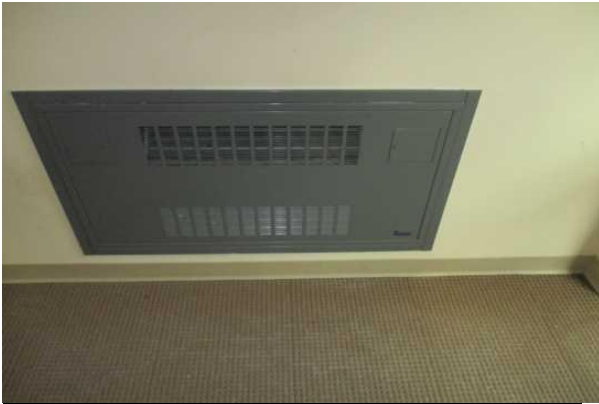
#43: FAN COIL UNIT, HYDRONIC
