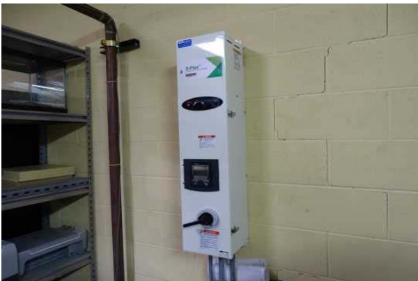
#29: VARIABLE FREQUENCY DRIVE (VFD)
