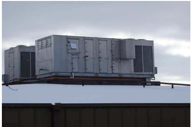
#34: PACKAGED UNIT (RTU)
