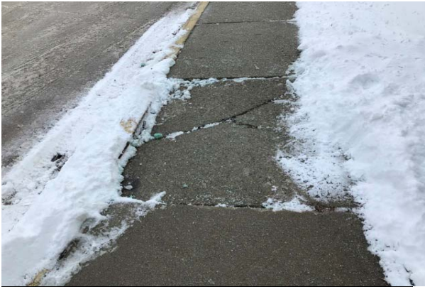
#7: SIDEWALK, TRIP HAZARD
