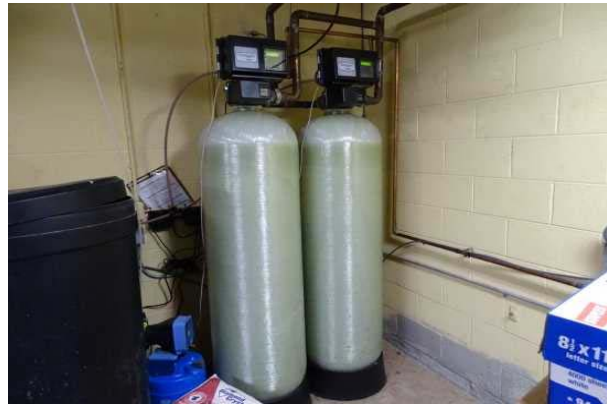
#28: WATER SOFTENING SYSTEM
