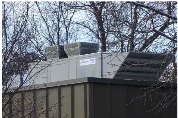
#36: MAKE-UP AIR UNIT
