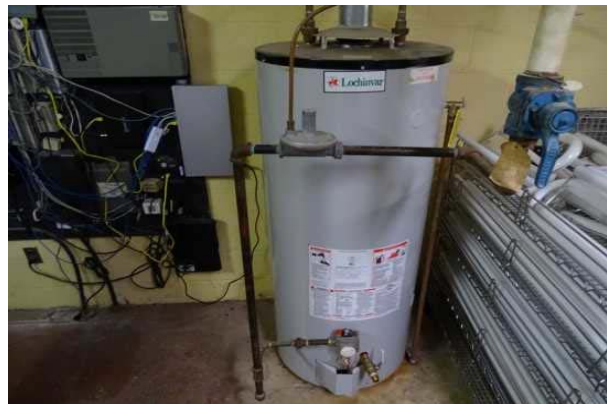
#30: WATER HEATER, GAS
