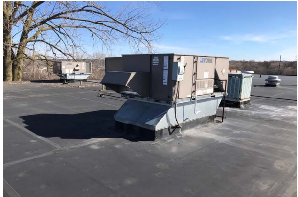
#22: TYPICAL PACKAGE UNIT (RTU)
