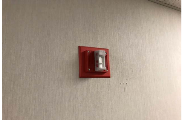
#28: FIRE ALARM STROBE
