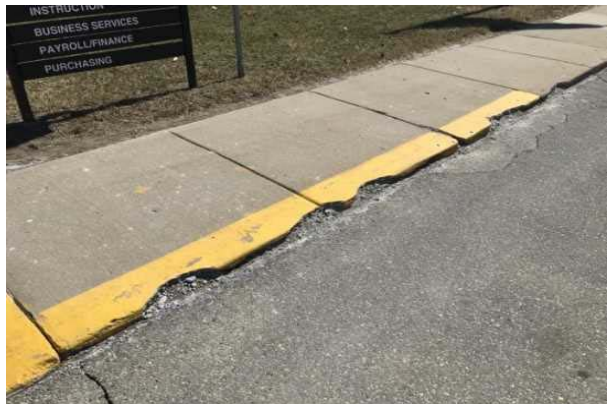
#36: DAMAGED CONCRETE SIDEWALKS
