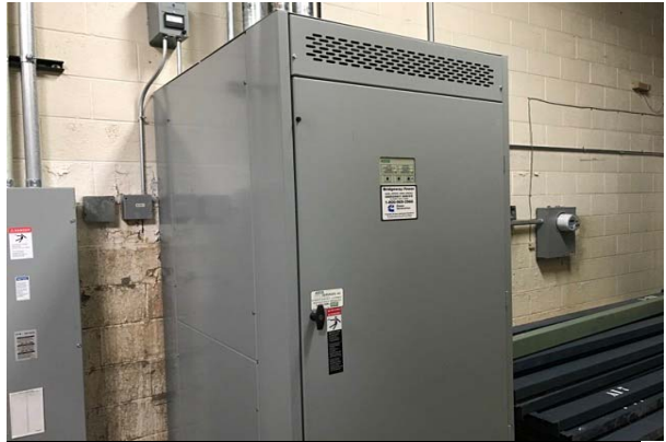
#32: EMERGENCY POWER AUTOMATIC TRANSFER SWITCH
