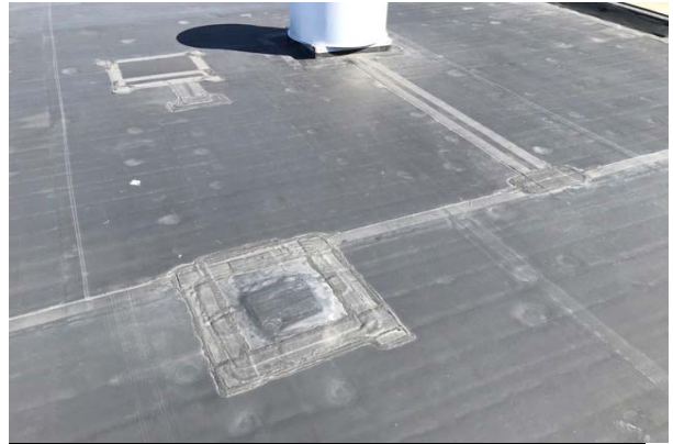
#8: PATCHED AREAS OF ROOF MEMBRANE
