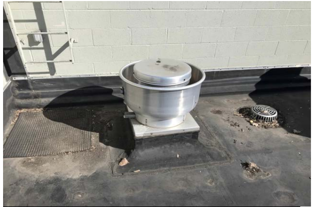
#26: TYPICAL EXHAUST FAN
