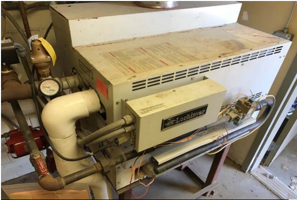
#25: GARAGE/LOADING DOCK AREA BOILER
