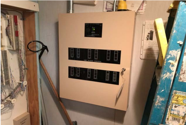
#27: CENTRAL FIRE ALARM PANEL
