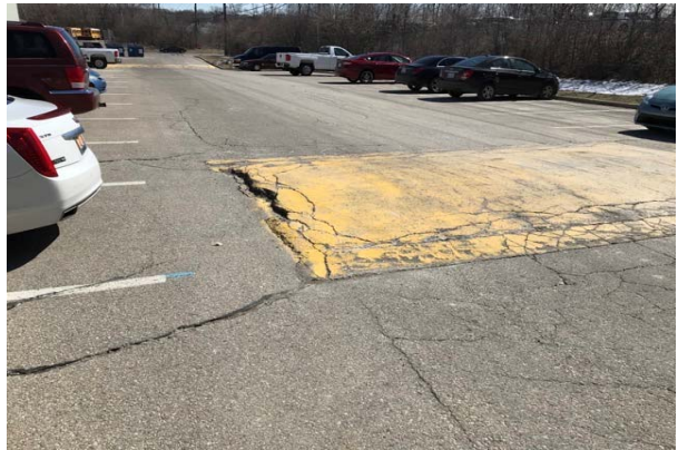
#34: DAMAGED PAVING AT SOUTH ELEVATION DRIVE AISLE
