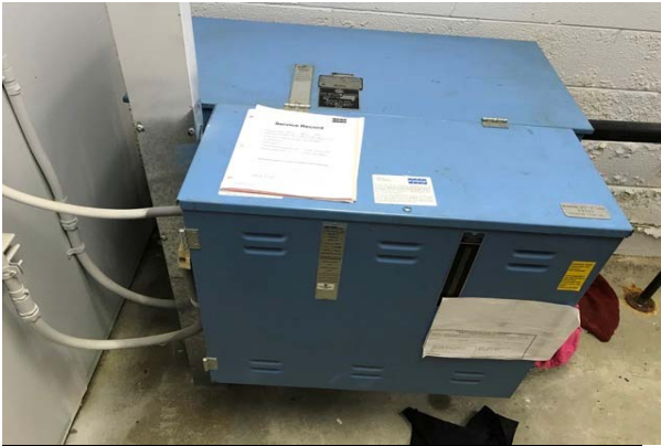
#19: HYDRAULIC ELEVATOR MACHINERY
