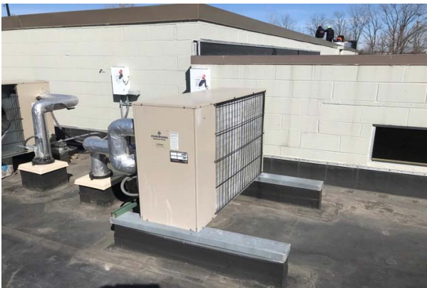
#23: COMPUTER ROOM AIR CONDITIONING (CRAC) UNIT
