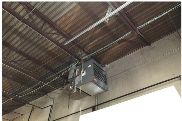
#24: WAREHOUSE SUSPENDED UNIT HEATER
