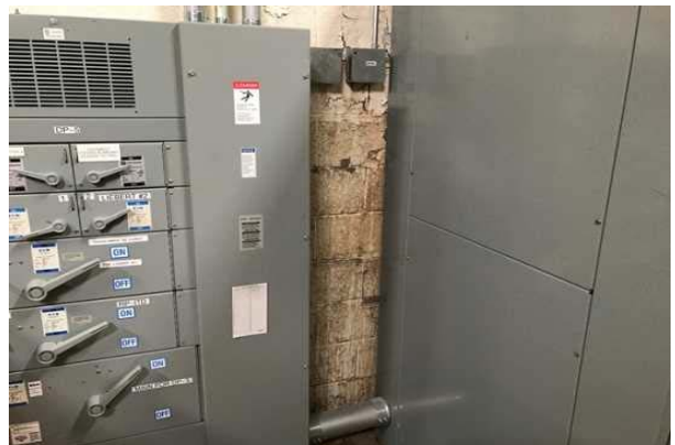
#10: WATER INFILTRATION AT EXTERIOR WALL
