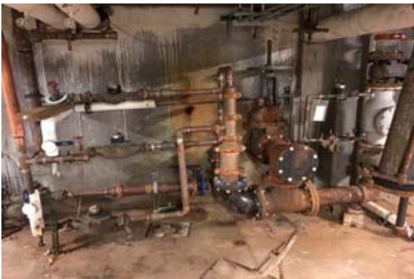
#47: PLUMBING SYSTEM, DOMESTIC SUPPLY
