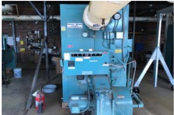
#40: HYDRONIC HEAT BOILER
