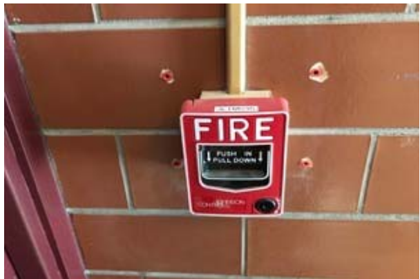
#60: MANUAL PULL STATION
