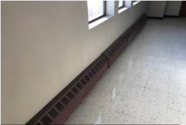
#43: RADIATOR, HYDRONIC BASEBOARD
