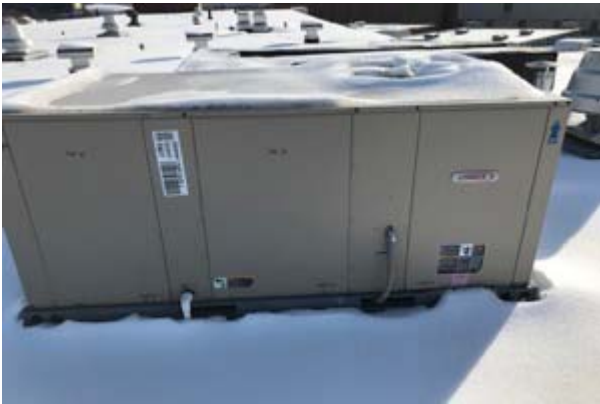
#39: ROOF TOP UNIT
