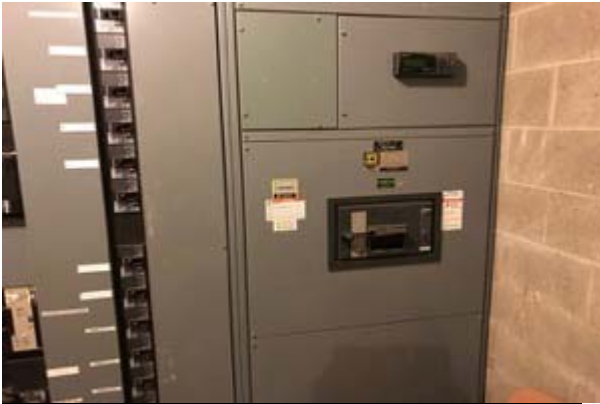
#55: 1200 AMP SWITCH GEAR
