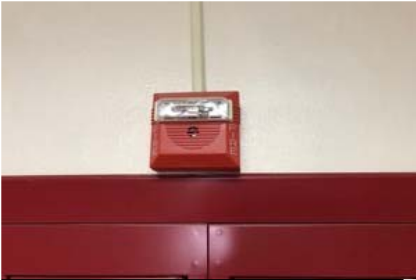
#61: FIRE ALARM DEVICE
