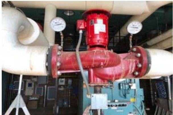
#46: HEAT DISTRIBUTION PUMP
