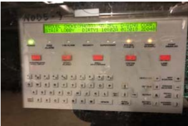
#65: BUILDING ADDRESSABLE FIRE ALARM PANEL
