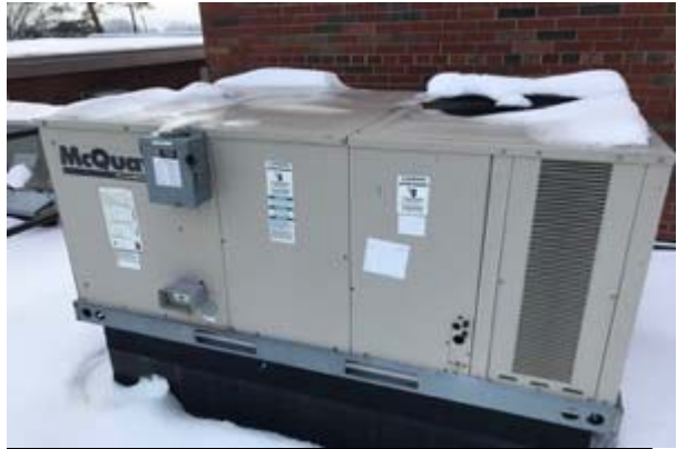
#38: ROOF TOP UNIT
