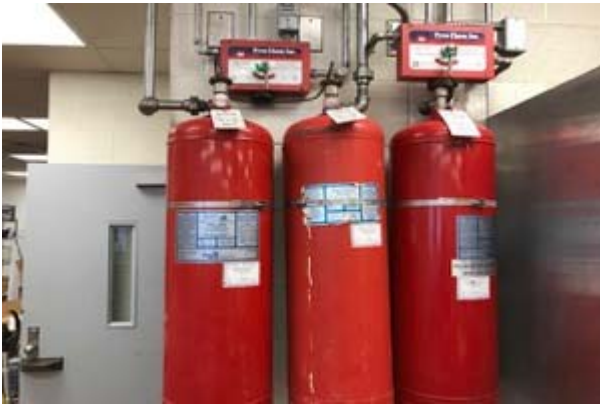
#63: FIRE SUPPRESSION SYSTEM
