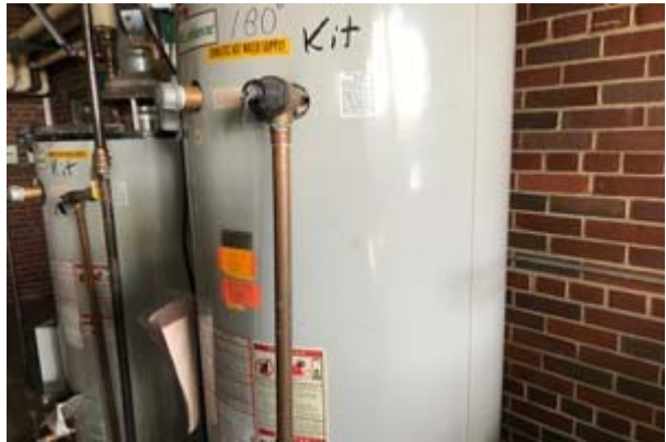
#52: KITCHEN DOMESTIC WATER HEATER
