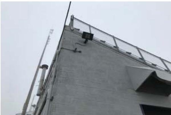
#17: EXTERIOR LED LIGHTING
