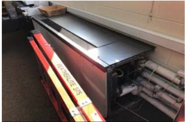
#44: HVAC SYSTEM HYDRONIC PIPING
