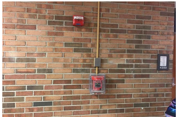
#58: FIRE ALARM SYSTEM
