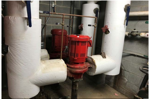
#26: DISTRIBUTION PUMP, HEATING WATER
