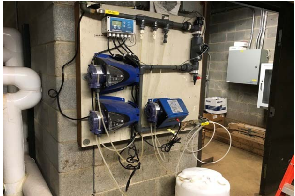
#40: CHEMICAL FEED SYSTEM
