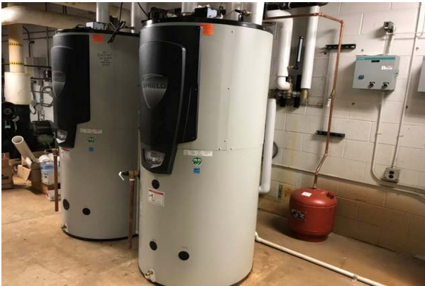
#27: DOMESTIC BOILER, GAS
