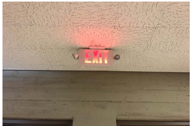
#48: EXIT LIGHTING FIXTURE, W/ BATTERY
