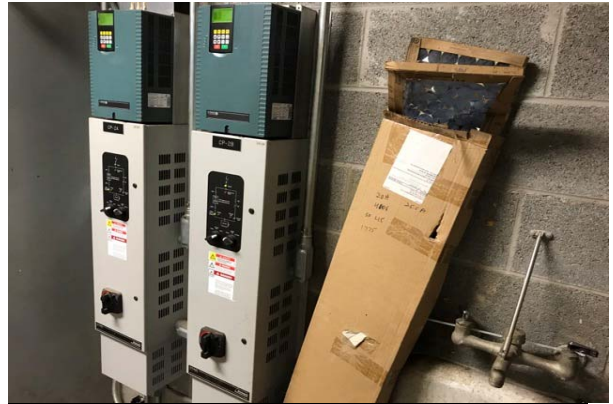
#56: VARIABLE FREQUENCY DRIVE (VFD)
