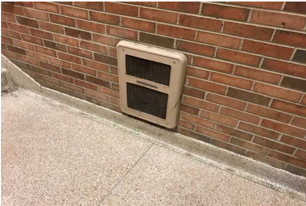
#45: WALL HEATER, GAS W/ ELECTRIC FAN
