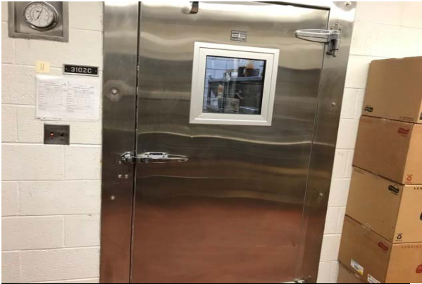
#67: COMMERCIAL KITCHEN, WALK-IN REFRIGERATOR
