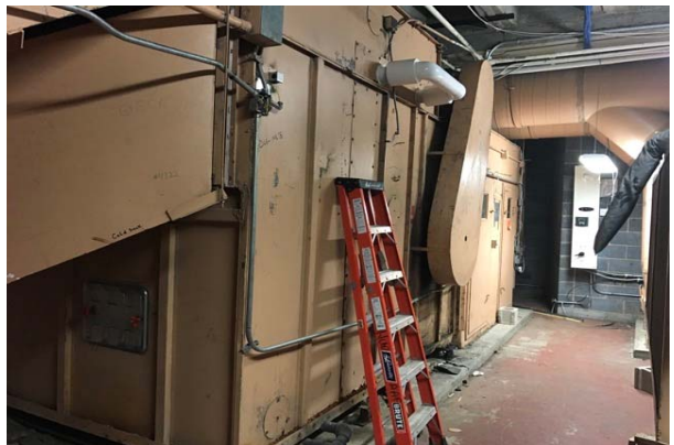
#36: AIR HANDLER UNIT
