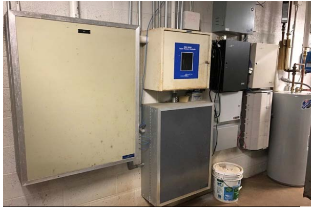
#38: BUILDING AUTOMATION SYSTEM (HVAC CONTROLS)
