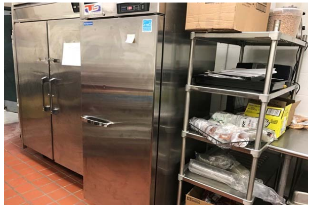
#64: COMMERCIAL KITCHEN, REFRIGERATOR
