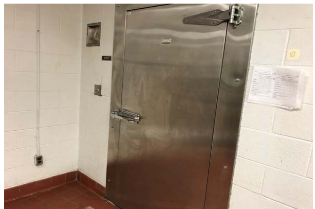
#66: COMMERCIAL KITCHEN, WALK-IN FREEZER
