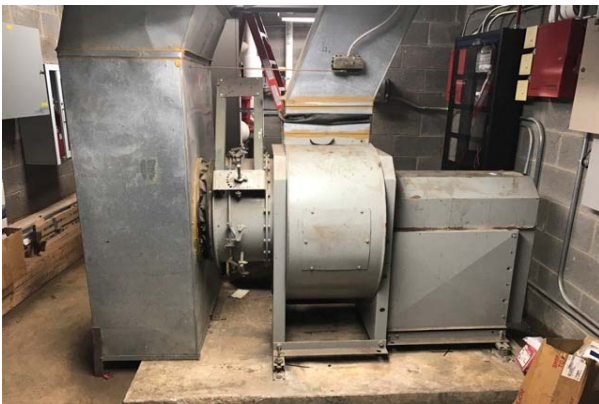
#41: EXHAUST FAN, CENTRIFUGAL
