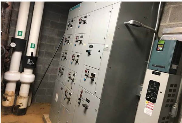
#53: MOTOR CONTROL CENTER
