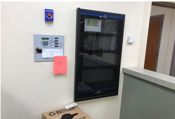
#57: FIRE ALARM CONTROL PANEL, ADDRESSABLE
