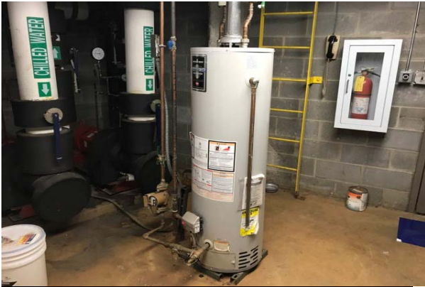
#31: WATER HEATER, GAS
