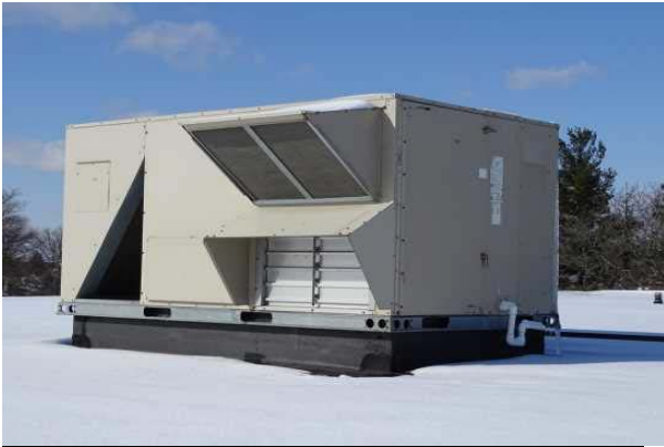
#31: PACKAGED UNIT (RTU)
