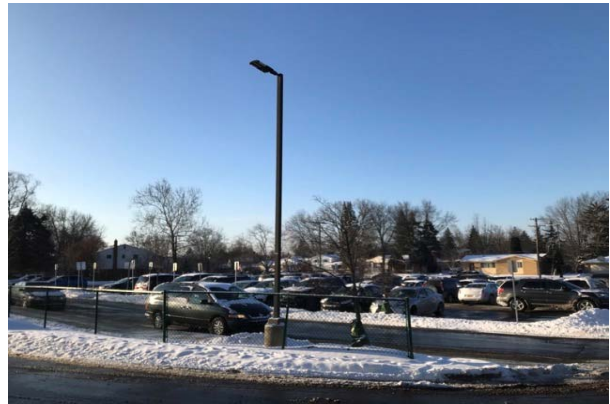
#16: EXTERIOR LIGHT POLE
