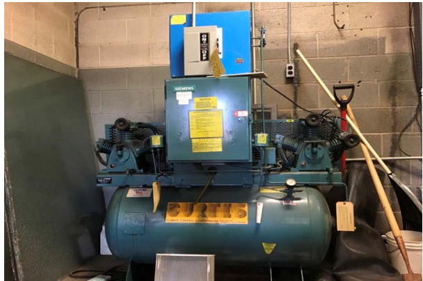
#28: AIR COMPRESSOR FOR PNEUMATICS
