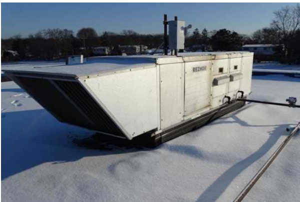
#29: MAKE-UP AIR UNIT
