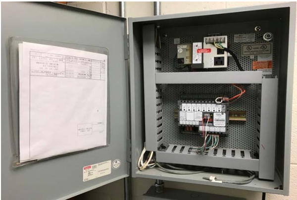
#27: BUILDING AUTOMATION SYSTEM (HVAC CONTROLS)
