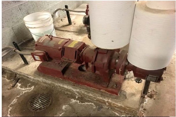
#26: HEATING WATER PUMP
