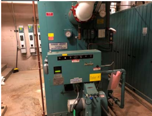
PHOTO #15: HVAC BOILER
