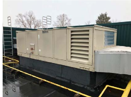
PHOTO #14: ROOFTOP UNIT
