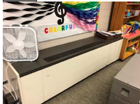
PHOTO #18: CLASSROOM UNIT VENTILATOR
