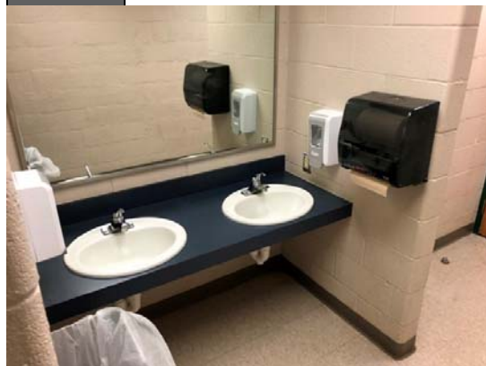
PHOTO #36: RESTROOM SINKS
