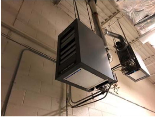
PHOTO #19: SUSPENDED UNIT HEATERS
