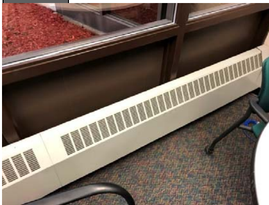
PHOTO #17: HYDRONIC TERMINAL UNIT
