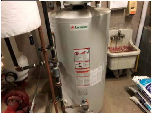
PHOTO #21: DOMESTIC WATER HEATER
