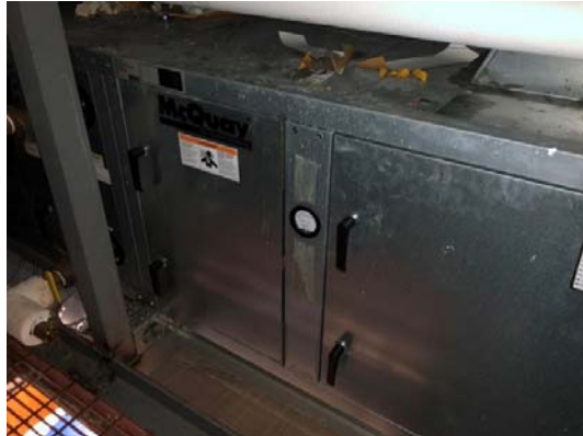
PHOTO #20: AIR HANDLER
