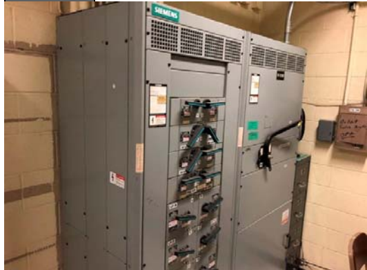
PHOTO #22: MAIN DISTRIBUTION PANEL
