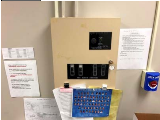
PHOTO #23: FIRE PANEL
