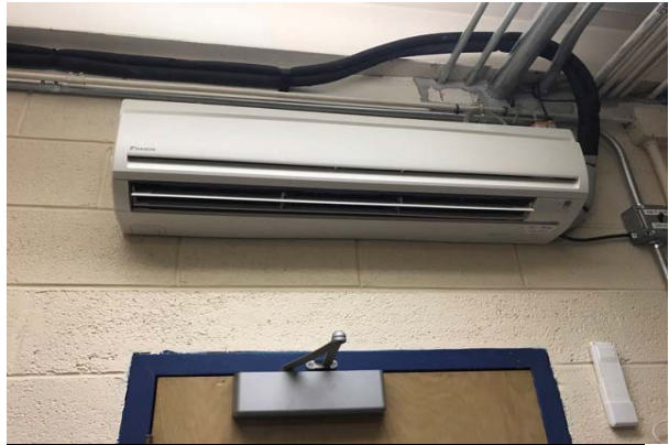
#26: DUCTLESS SPLIT SYSTEM
