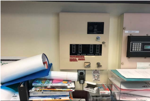
#37: FIRE ALARM CONTROL PANEL
