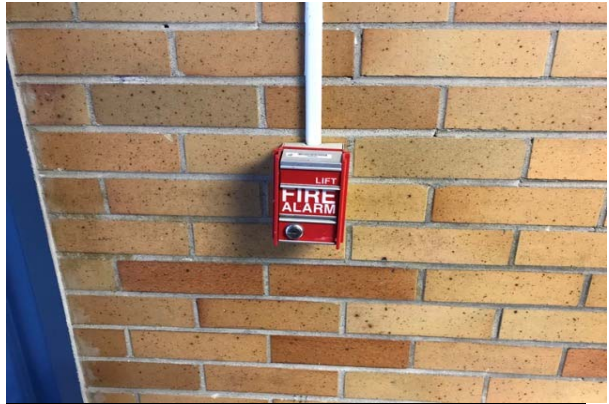
#38: FIRE ALARM SYSTEM, SCHOOL
