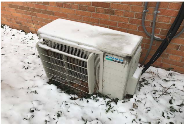
#29: DUCTLESS SPLIT SYSTEM
