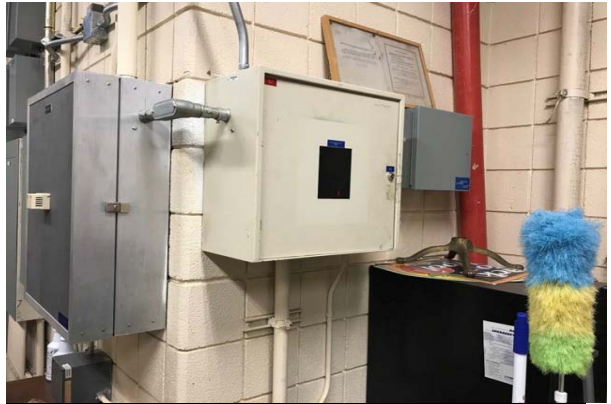
#32: BUILDING AUTOMATION SYSTEM (HVAC CONTROLS)
