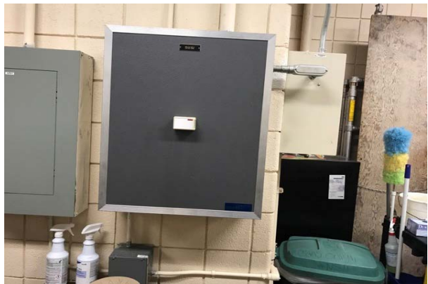
#30: BUILDING AUTOMATION SYSTEM (HVAC CONTROLS)
