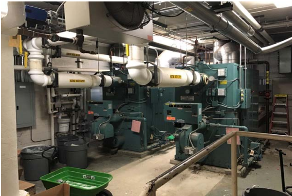
#33: CENTRAL HEATING SYSTEM
