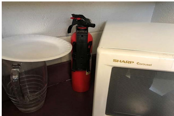
#18: NON-CERTIFIED FIRE EXTINGUISHER
