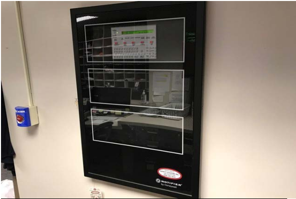
#43: FIRE ALARM CONTROL PANEL
