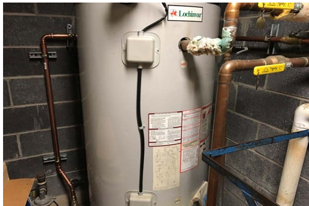
#36: COMMERCIAL WATER HEATER
