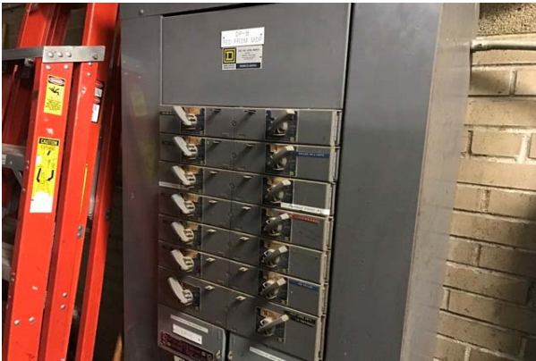
#39: MOTOR CONTROL CENTER
