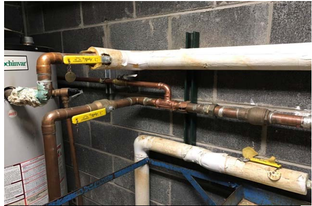
#38: WATER PIPING SYSTEM, DOMESTIC WATER SUPPLY
