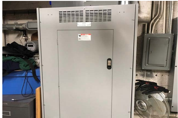
#40: MAIN DISTRIBUTION PANEL
