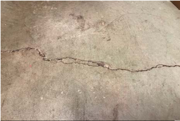
#7: CRACKED CONCRETE SLAB-ON-GRADE
