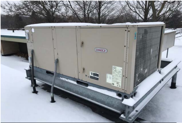
#13: PACKAGED UNIT (RTU),
