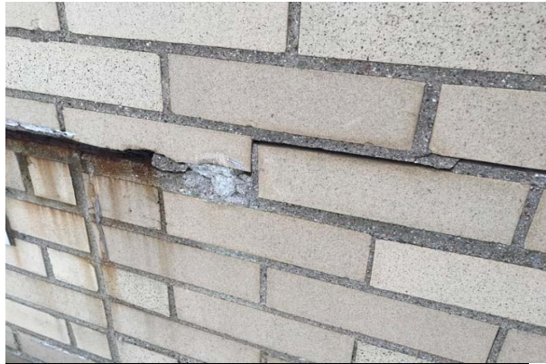
#14: BRICK VENEER CRACKING
