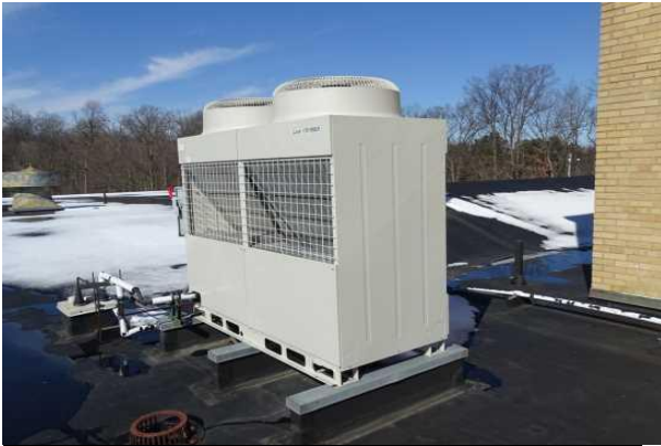
#55: SPLIT SYSTEM, CONDENSING UNIT
