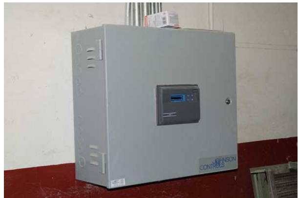
#58: BUILDING AUTOMATION SYSTEM (HVAC CONTROLS),
