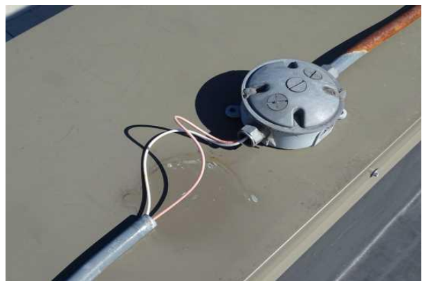
#60: EXPOSED WIRING ON ROOF
