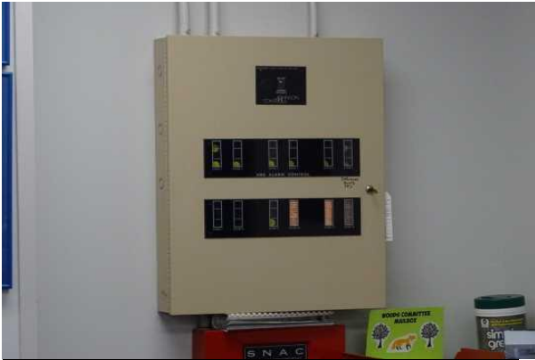
#61: FIRE ALARM PANEL
