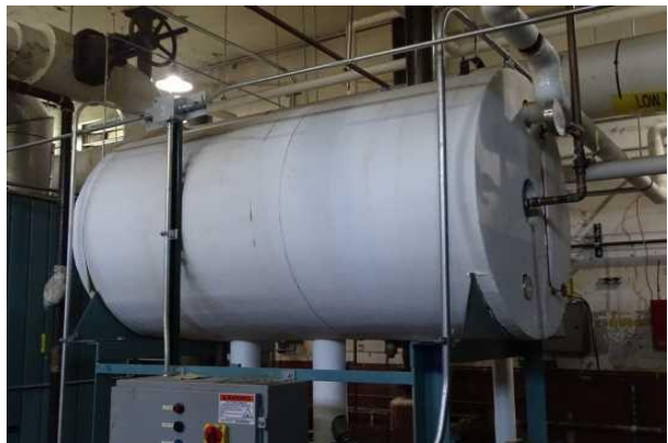
#48: CONDENSATE RETURN STATION
