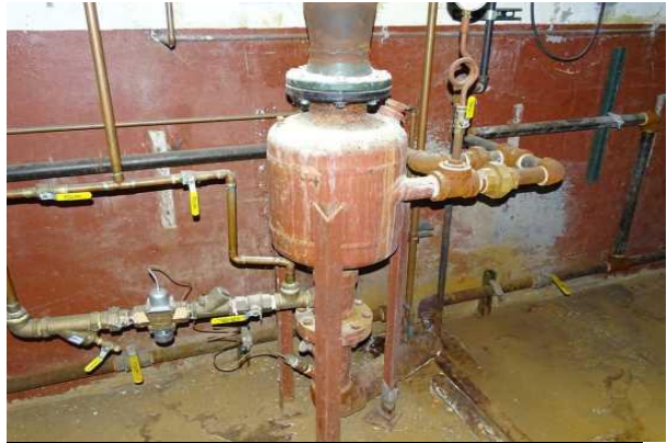
#44: BOILER BLOWDOWN SYSTEM
