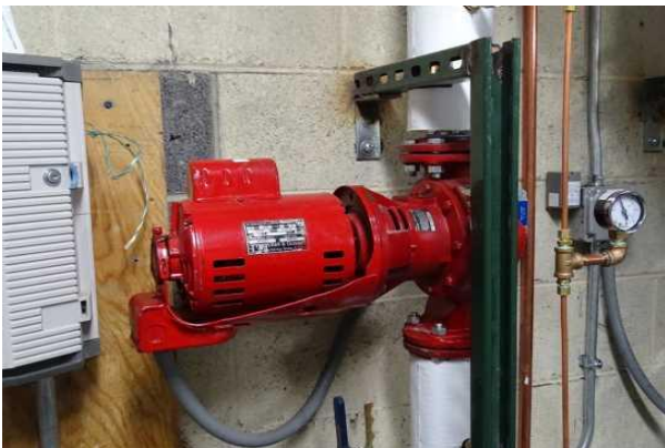
#41: DISTRIBUTION PUMP, HEATING WATER
