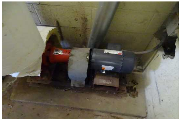
#42: DISTRIBUTION PUMP, HEATING WATER
