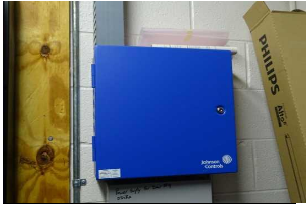
#32: BUILDING AUTOMATION SYSTEM HYBRID
