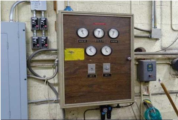
#31: BUILDING AUTOMATION SYSTEM HYBRID
