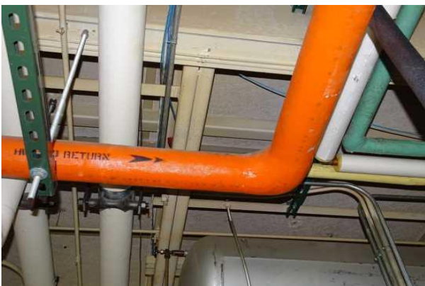
#29: PIPING POSSIBLE ASBESTOS
