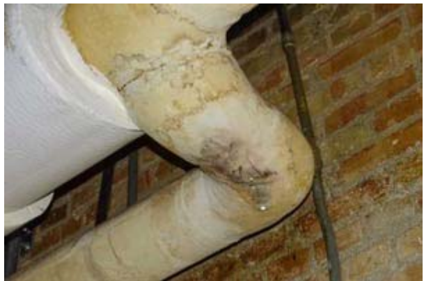
#54: POSSIBLE ASBESTOS CONTAINING MATERIAL
