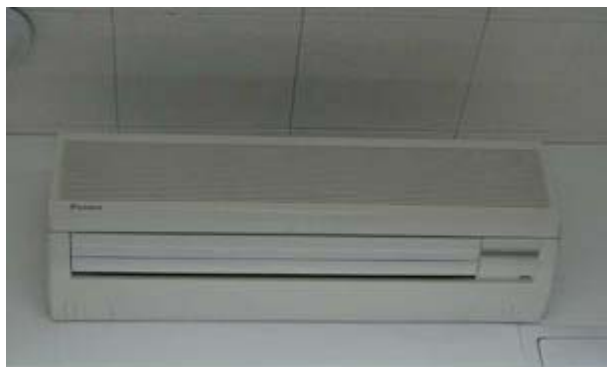
#78: DUCTLESS SPLIT SYSTEM
