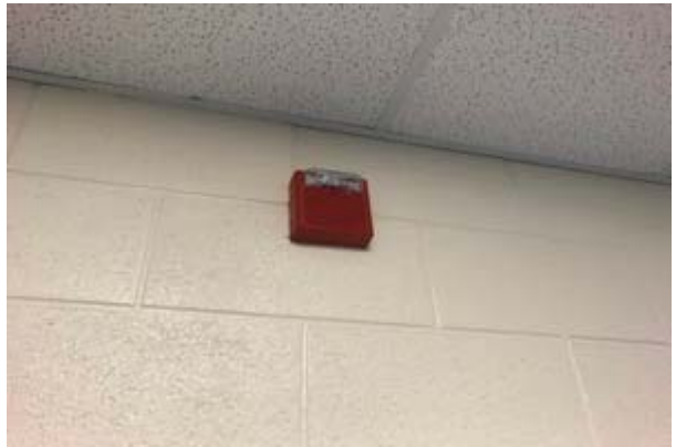
#88: FIRE ALARM HORN
