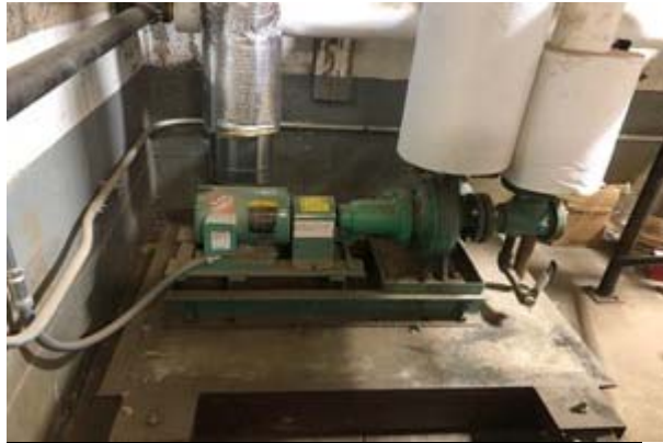
#62: HEATING WATER PUMP
