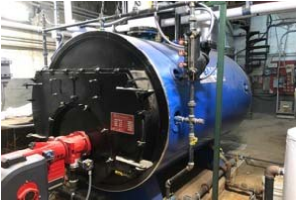
#73: LOW PRESSURE STEAM BOILER
