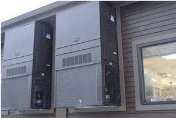
#61: SOUTH ANCILLARY STRUCTURE, PACKAGED TERMINAL AIR CONDITIONER
