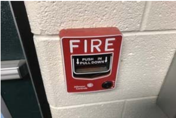
#87: MANUAL PULL STATION
