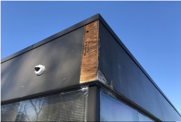
#7: ALUMINUM SIDING, REPLACE
