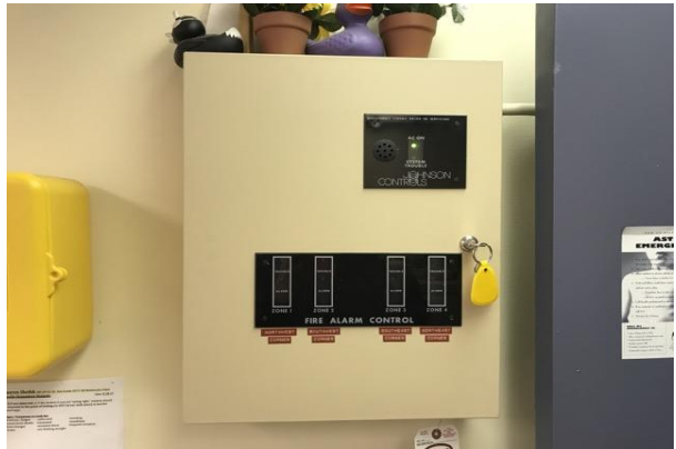
#10: FIRE ALARM PANEL, REPLACE
