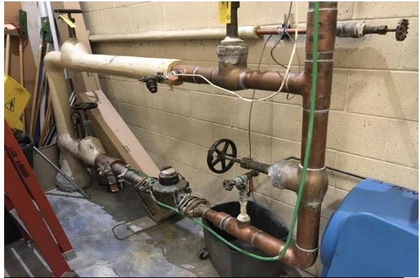
#20: DISTRIBUTION PIPING, DOMESTIC WATER SUPPLY
