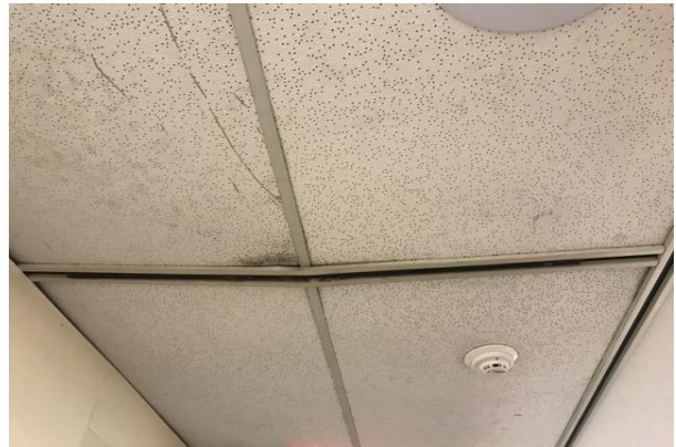
#46: SUSPENDED ACOUSTICAL CEILING TILE (ACT), REPLACE
