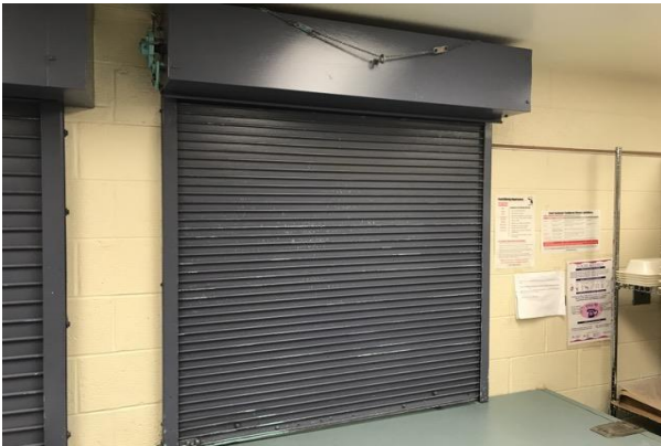
#45: ROLL-UP DOOR, REPLACE
