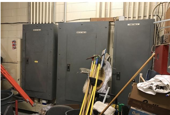
#41: MAIN DISTRIBUTION PANELS
