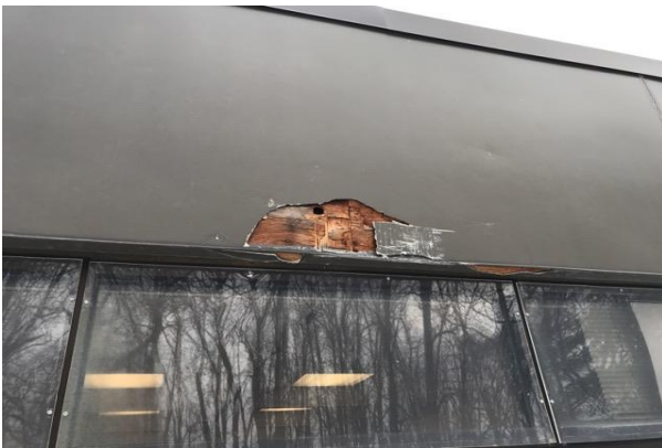
#21: ALUMINUM SIDING, REPLACE
