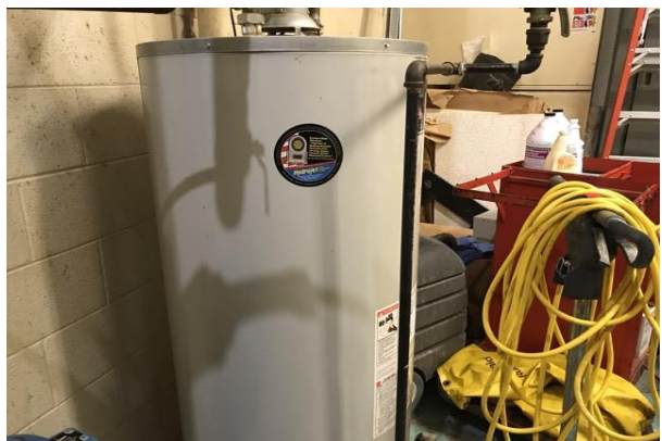
#24: WATER HEATER, COMMERCIAL, GAS
