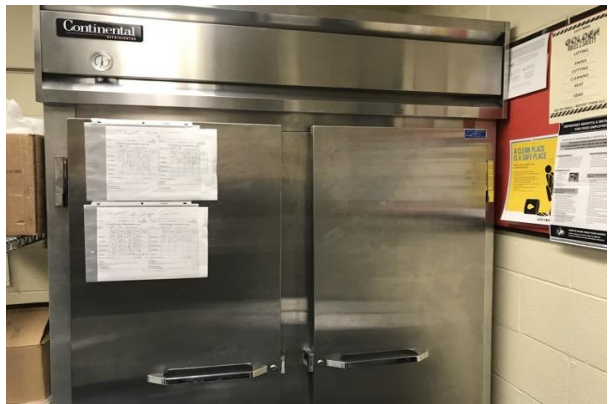
#12: REACH-IN REFRIGERATOR, REPLACE
