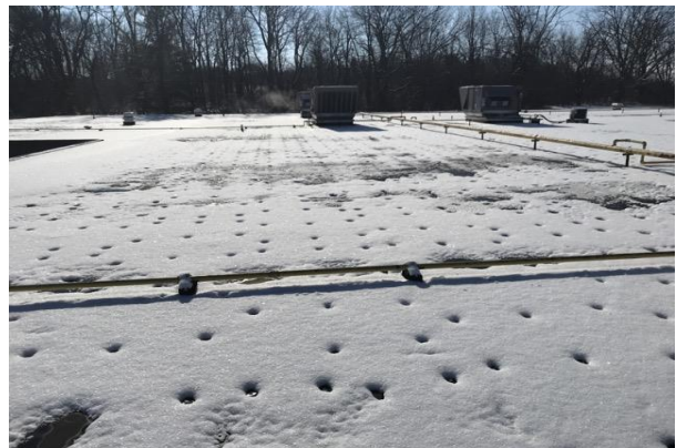
#18: ROOF, BUILT-UP MEMBRANE, REPLACE
