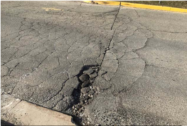
#49: CRACKED AND DAMAGED PAVING AT DRIVE AISLE
