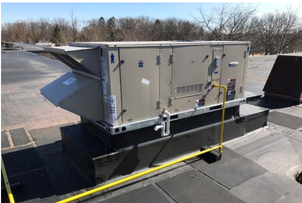
#35: TYPICAL GAS-FIRED PACKAGE UNIT (RTU)
