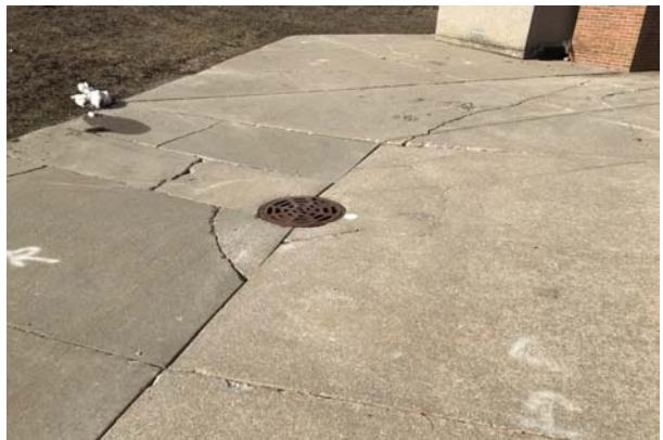
#52: CRACKED CONCRETE SIDEWALK
