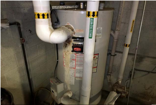
#31: DOMESTIC WATER HEATER
