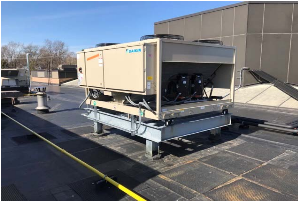
#33: AIR-COOLED CONDENSING UNIT CONNECTED TO PENTHOUSE AHU
