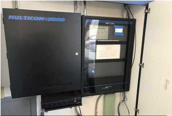
#43: FIRE ALARM CONTROL PANEL
