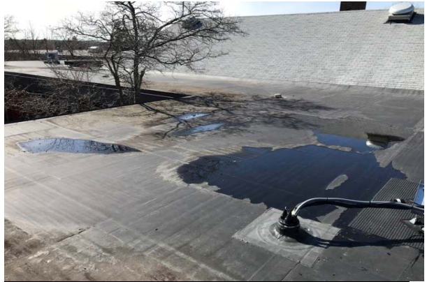
#8: FLAT ROOF, ISOLATED MINOR PONDING
