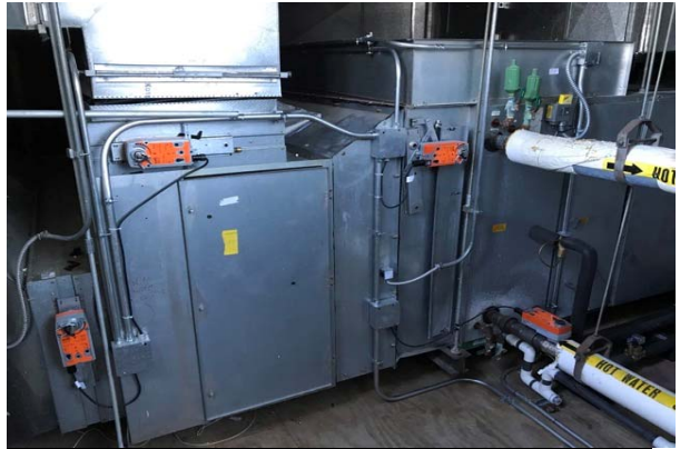
#32: PENTHOUSE AIR HANDLER
