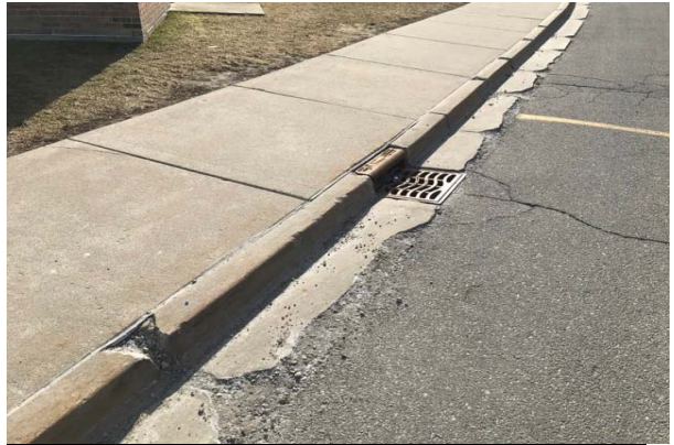
#50: CONCRETE CURB DAMAGE
