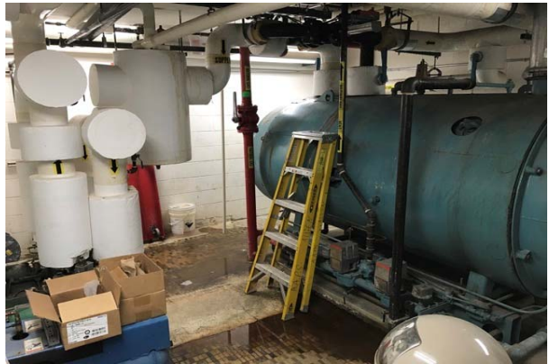
#28: BOILER ROOM B
