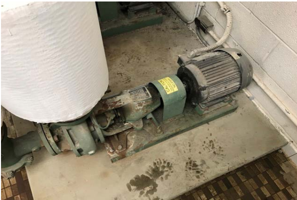
#39: DISTRIBUTION PUMP, HEATING WATER
