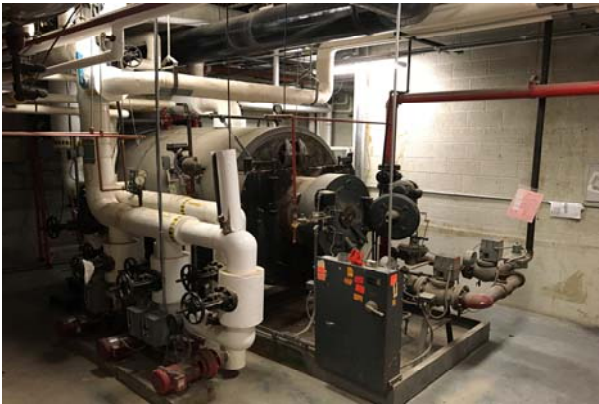
#27: BOILER ROOM A
