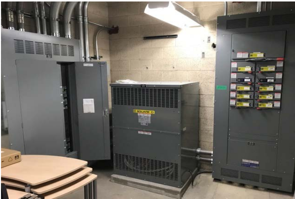
#45: MAIN ELECTRICAL COMPONENTS
