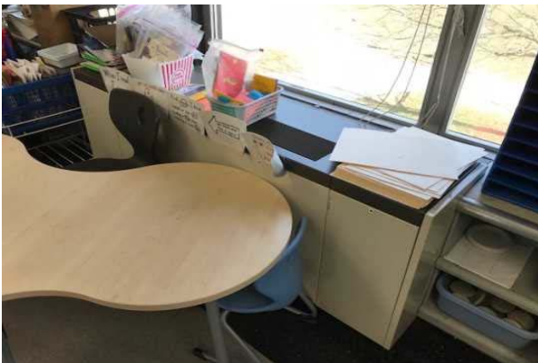
#41: TYPICAL CLASSROOM UNIT VENTILATOR
