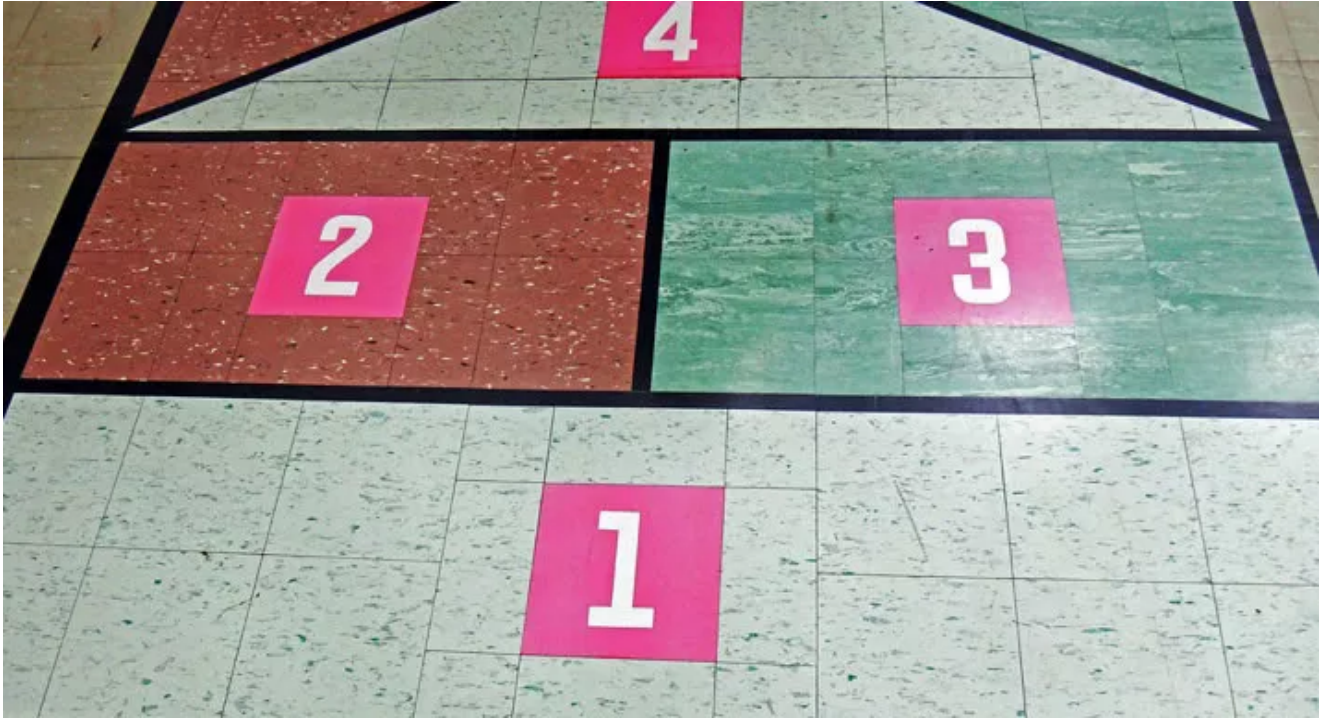
This asbestos-containing floor tile was used as a hopscotch game in an elementary school gymnasium.
