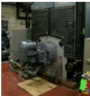
Figure 2: H.B. Smith Boiler at Assunpink
