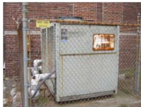
Figure 2: Trane chiller serving new portion of Health Careers
