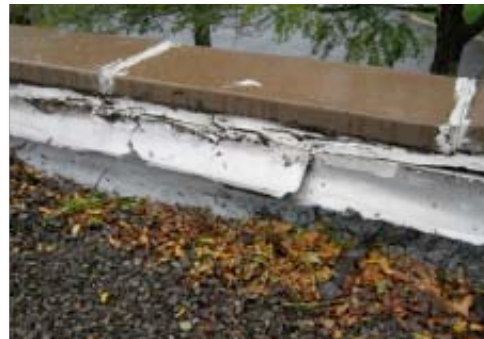
Figure 3: In some areas concrete slabs have fallen and have been replaced
