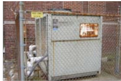
Figure 2: Trane chiller serving new portion of Health Careers
