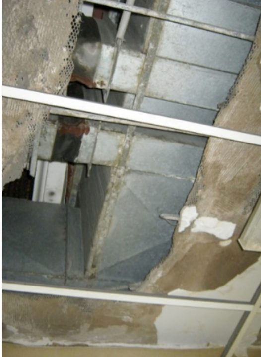
Figure 1: Roof damage causes further damage to ceiling and HVAC equipment
