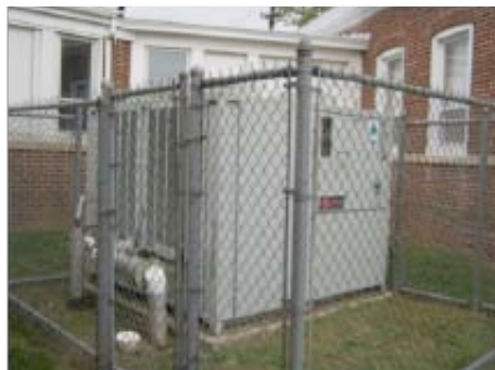
Figure 1: Trane chiller serving original portion of Health Careers
