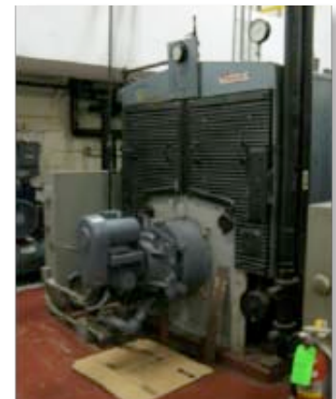
Figure 1: Typical gas-fired boiler at the Assunpink Center
