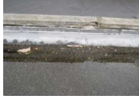
Figure 2: Concrete roof-edge slabs which are not secure due to degradation
