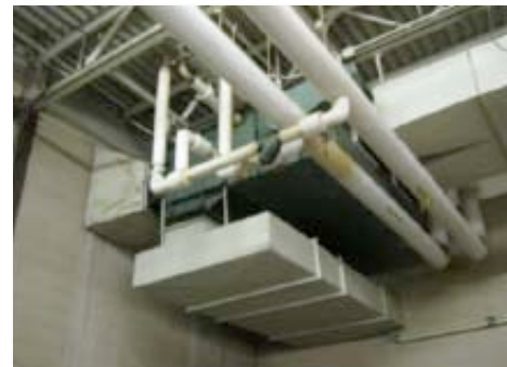
Figure 1: Heating and Ventilating unit common throughout the Assunpink and Sypek Campuses
