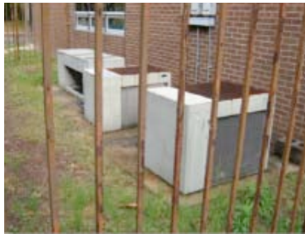
Figure 1: Cooling equipment serving portions of C Annex at the Sypek Center.
