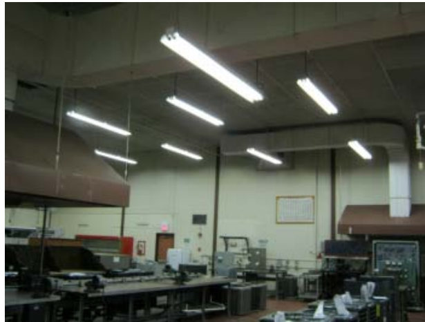
Figure 4: Two-lamp 8 ft. T12 fixtures common in Shop Areas
