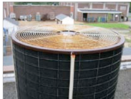
Figure 3: Equipment was found to be in poor condition
