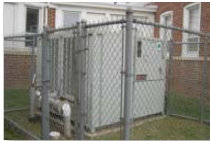
Figure 1: Trane chiller serving original portion of Health Careers
