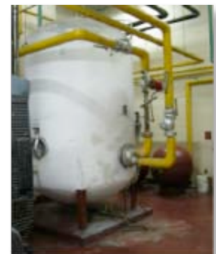
Figure 1: 2,115 gallon DHW storage tank at Sypek Center
