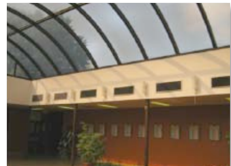
Figure 6: Central Court at Sypek Building C where excessive heat gain occurs
