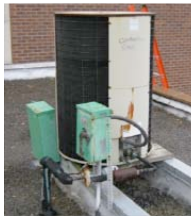
Figure 2: Split system common at the Assunpink and Sypek campuses
