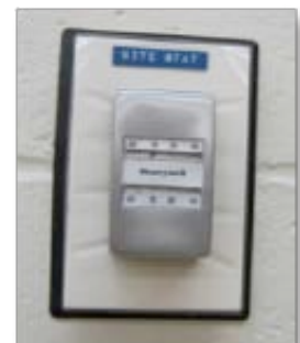
Figure 2: The position of “Night” thermostats currently control the unoccupied temperature setpoints in each space
