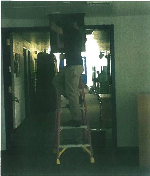
Significant infrastructure and electrical work has been completed to support the use of the new technology.
