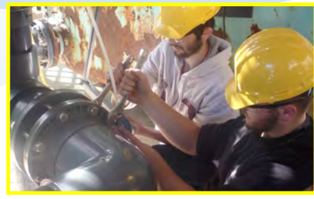
INTERNSHIP: STC Plumbing students assist Pottsville City with new piping installations at the JFK pool.
