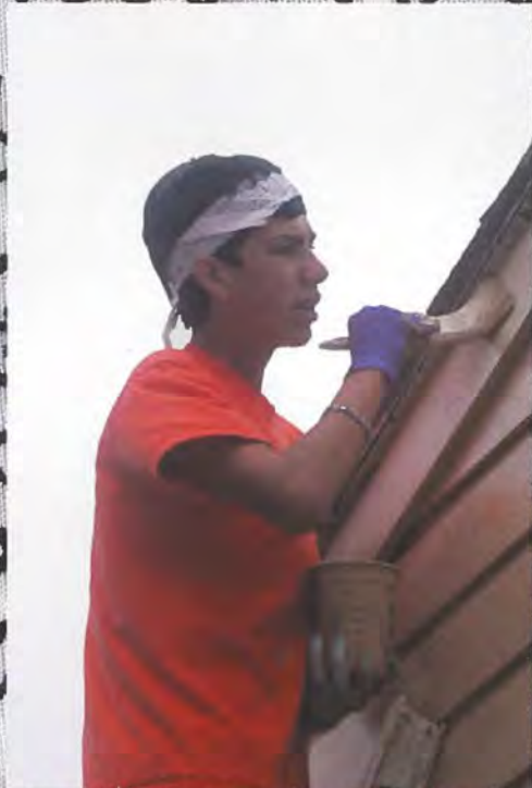
Sophomore JD Longoria paints the roof of a house after climbing the ladder to reach the top.
