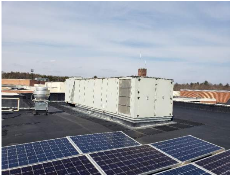
High School Cafeteria RTU-7
