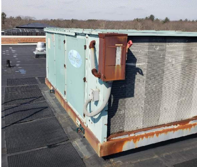
Packaged Roof Top Unit, RTU-36
