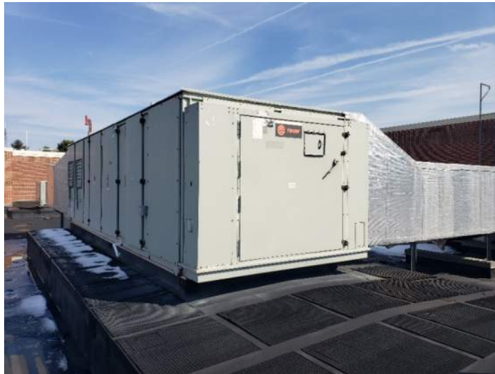
Middle School Gym Heating and Ventilation Unit, RTU-3
