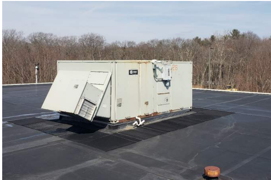
Administration Office Area RTU-26
