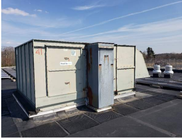
Packaged Roof Top Unit, RTU-41
