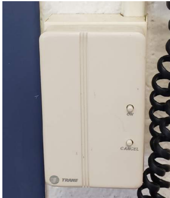
Typical Classroom Thermostat
