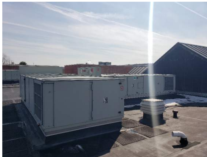
Middle School Music Heating and Ventilation Units, RTU-8 and RTU-9
