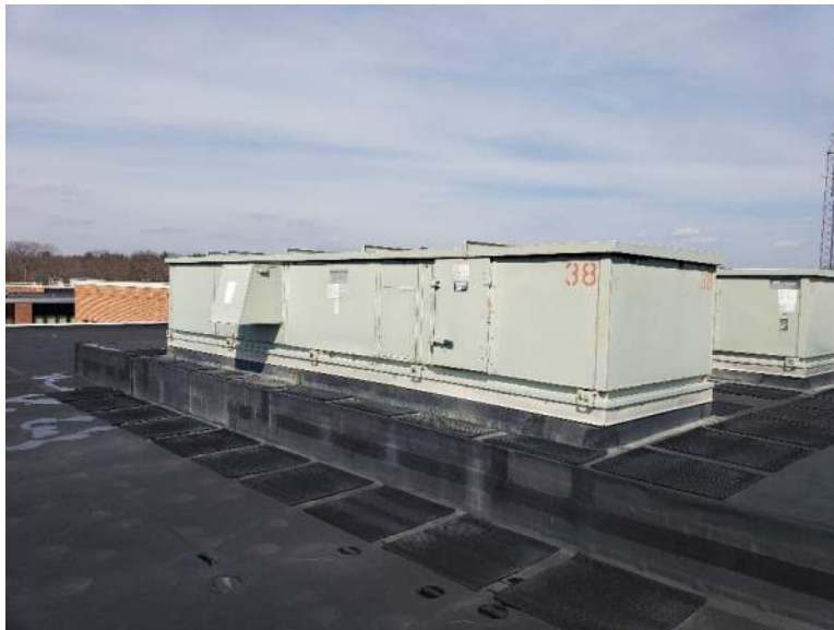
100% Outside Air Unit, RTU-38
