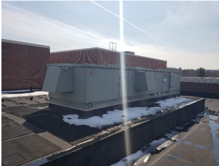
Locker Rooms Heating and Ventilation Unit, RTU-4
