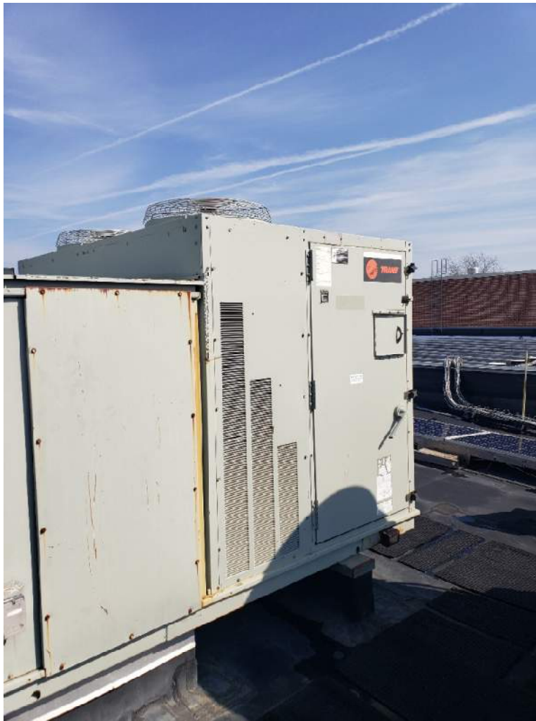
Middle School Cafeteria, RTU-5
