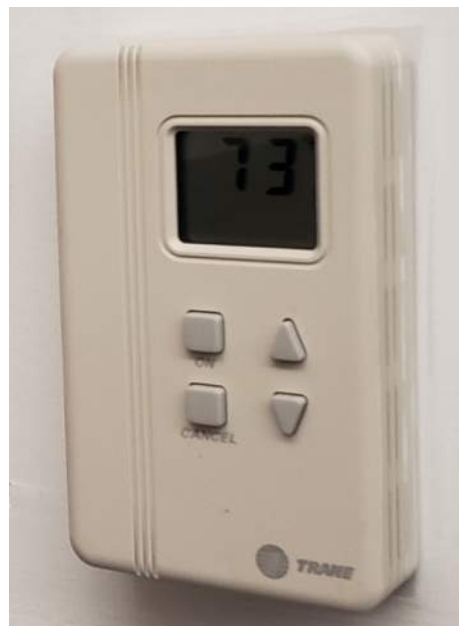
Typical Office Thermostat
