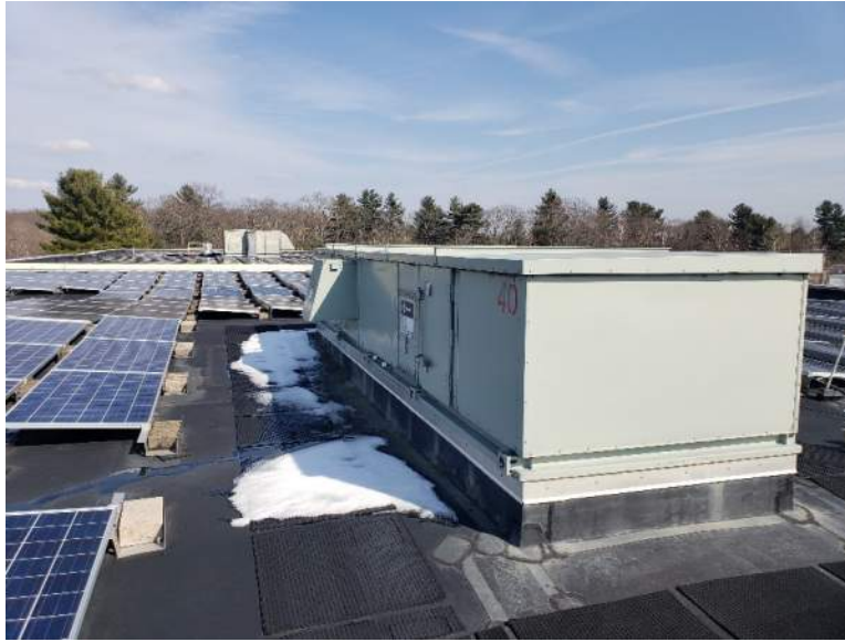
100% Outside Air RTU-40
