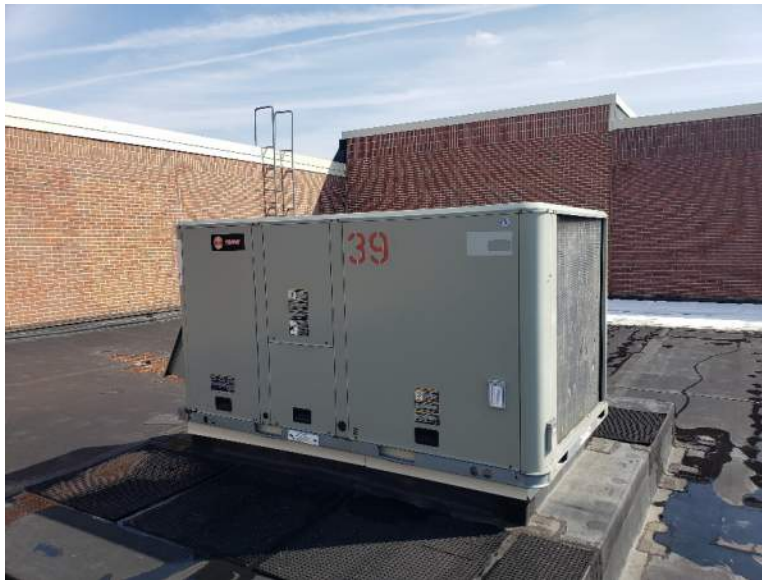
Typical Packaged Roof Top Unit, RTU-39
