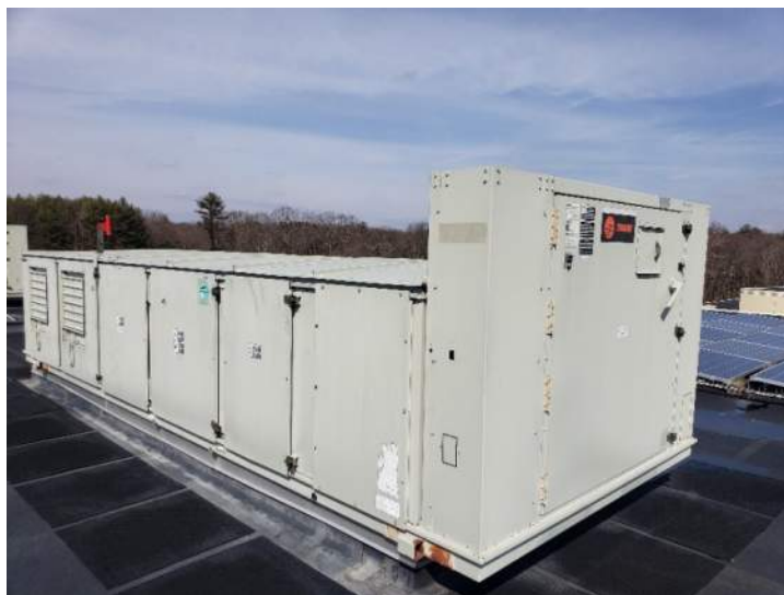
Gym Heating and Ventilation Unit RTU-12
