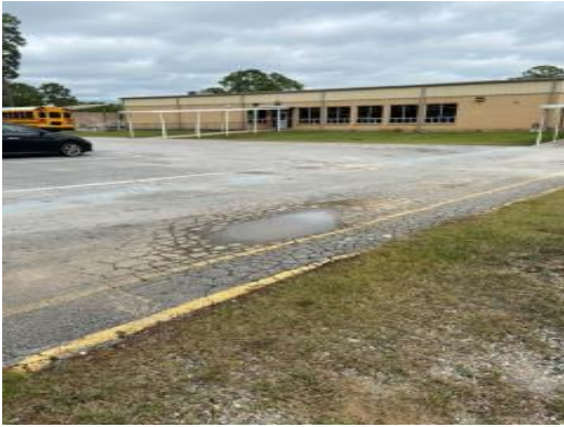
Failing asphalt in west parking area
