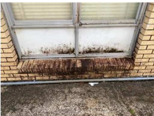
Dirty window sills
