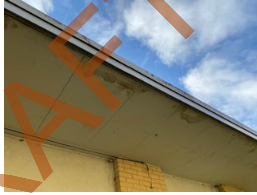
Water damaged soffit paneling
