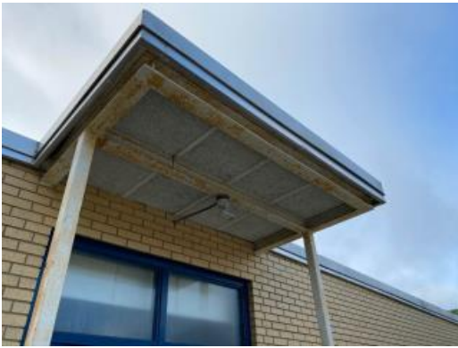
Rusted canopy and structure
