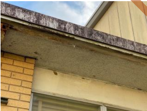
Dirty coping and rusted metal soffit trim
