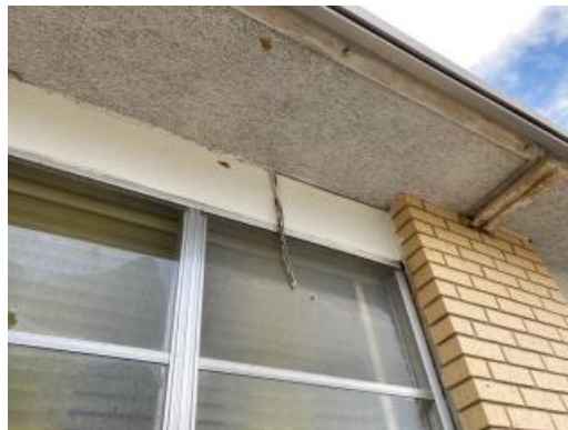
Failing caulk joints
