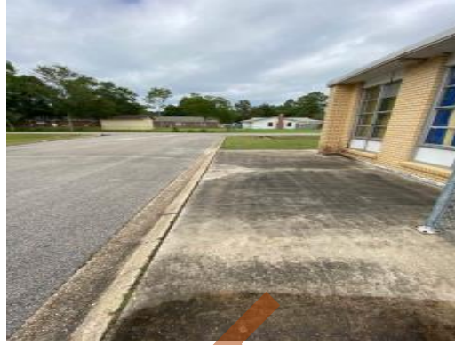
Sidewalk failure to the west of the northeast wing
