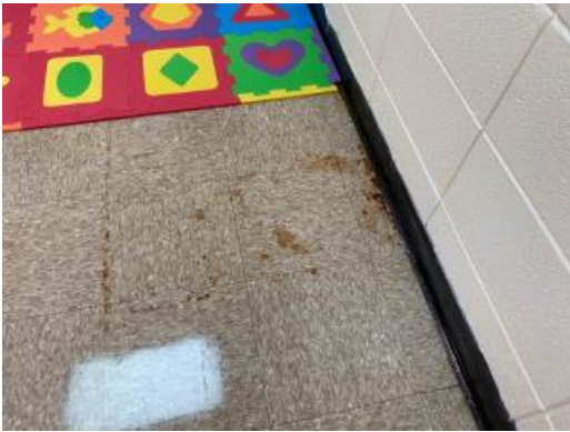
Stained and peeling VCT
