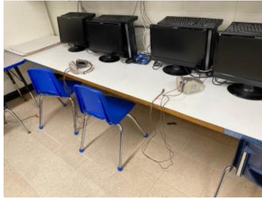
Peeling veneer at classroom casework
