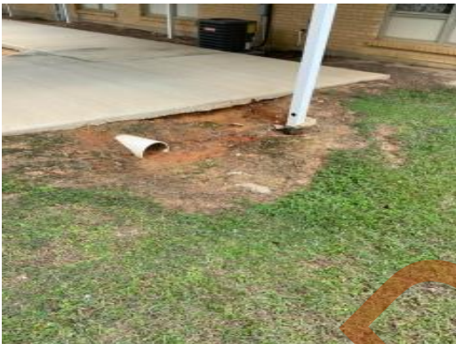
Sidewalk to west parking lot being undermined
