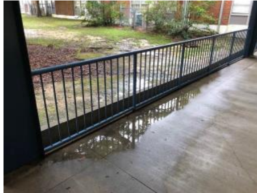
Water ponding north of breezeway
