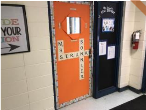
Classroom door hardware not ADA compliant
