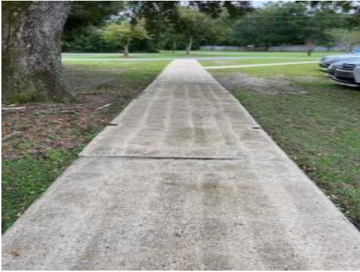
Concrete sidewalk buckling
