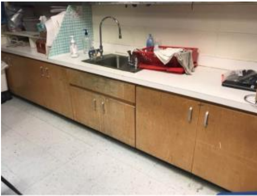
Worn classroom cabinetry
