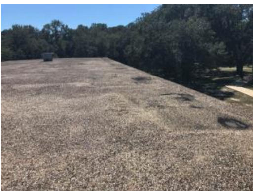
Built up roofing with evidence of leaks
