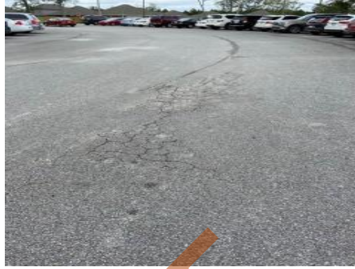
Cracked asphalt pavement
