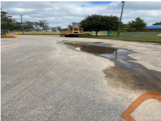
Ponding in east parking lot
