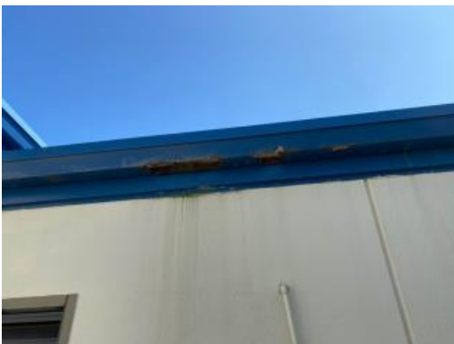
Rusted out gutters
