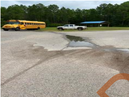
Driveway pavement failure
