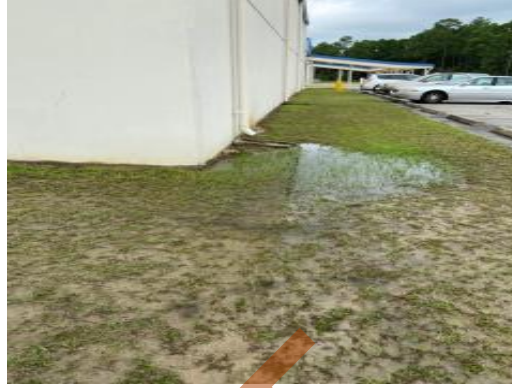
Area around southeast building corner ponding
