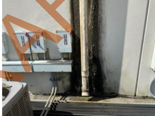
Area around downspout to be cleaned
