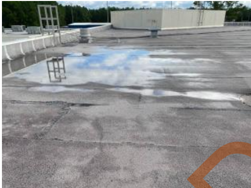
Ponding on roof
