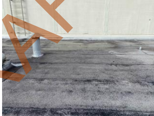
Bubbled and blistered roof
