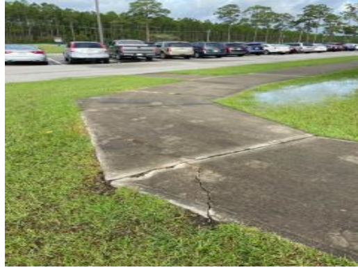
Damaged south sidewalk
