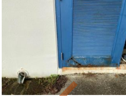
Rusted exterior metal door
