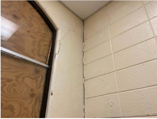
Crack at ticket booth area
