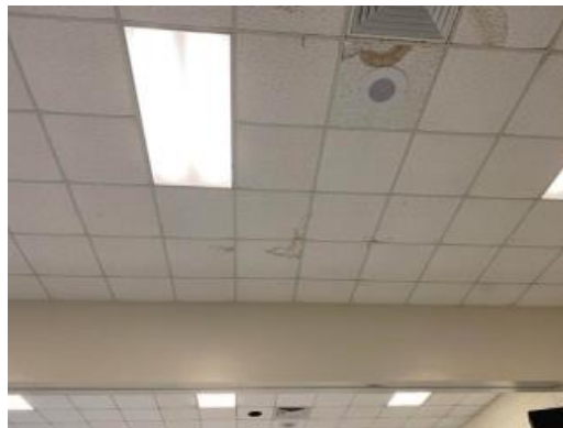
Water damaged ceiling tiles
