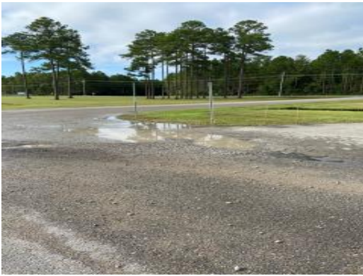
Failing asphalt at southwest corner of west parking lot
