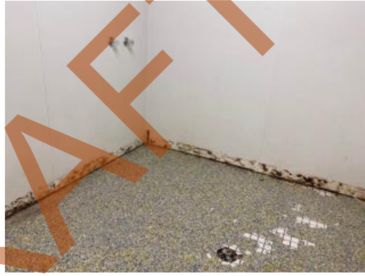
Damaged wall in group shower area
