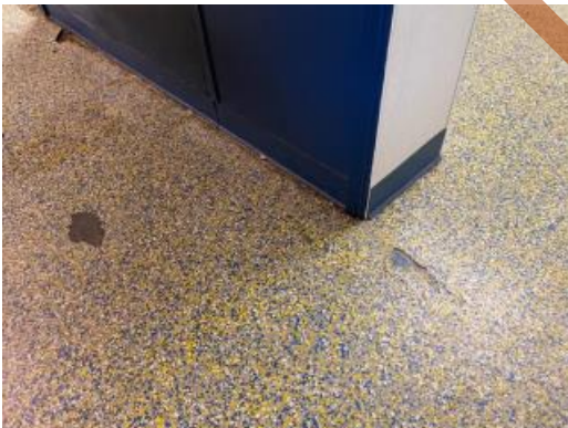
Peeling epoxy flooring
