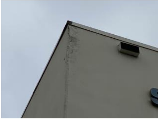
Deteriorating precast panel on west side of building
