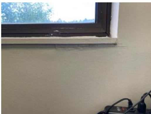
Water damage at leaking window
