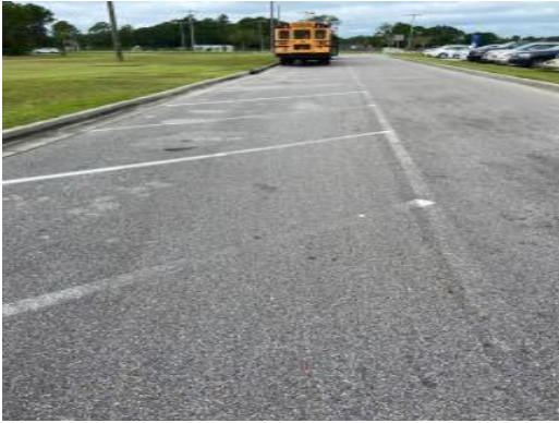
Faded parking striping on the south drive
