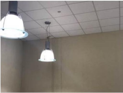
Roof leak north stairwell
