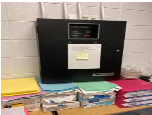
Obsolete fire alarm system
