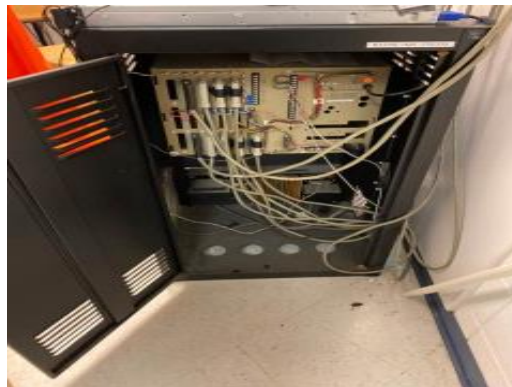
Obsolete PA system
