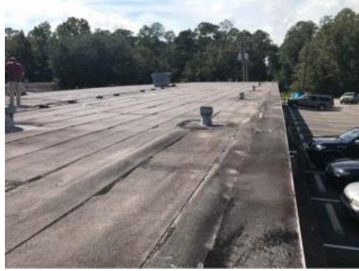
Delaminating mod bit roof
