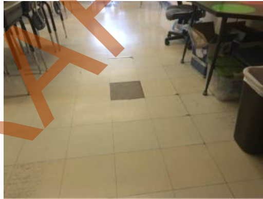
Missing and chipped VCT
