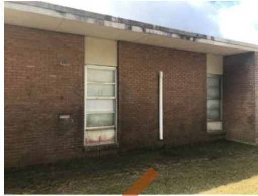
Building A old worn windows
