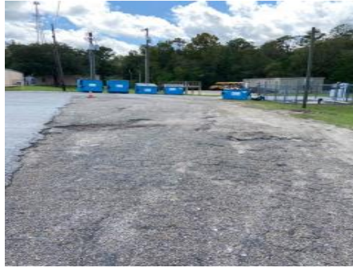
Failed asphalt west of cafeteria
