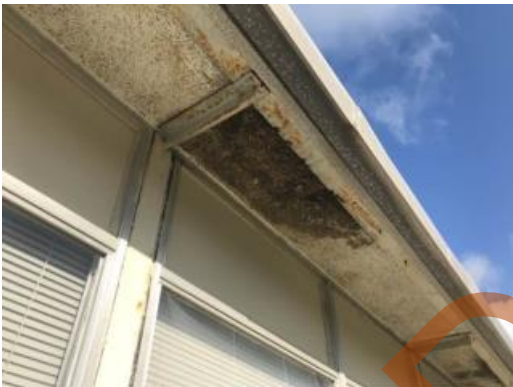
Building A soffit damage
