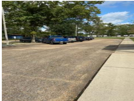
Damaged asphalt north of main entry
