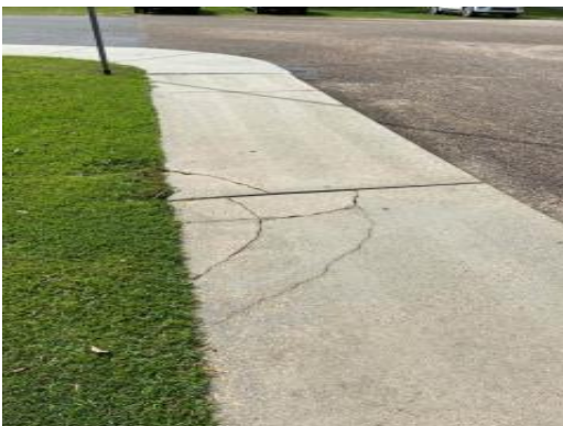
Cracked sidewalk by the main entrance
