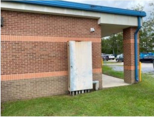
Corroded electrical panel
