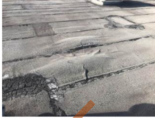
Aged and bubbled roofing
