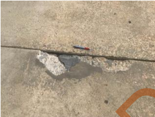
Damaged sidewalk south of gym
