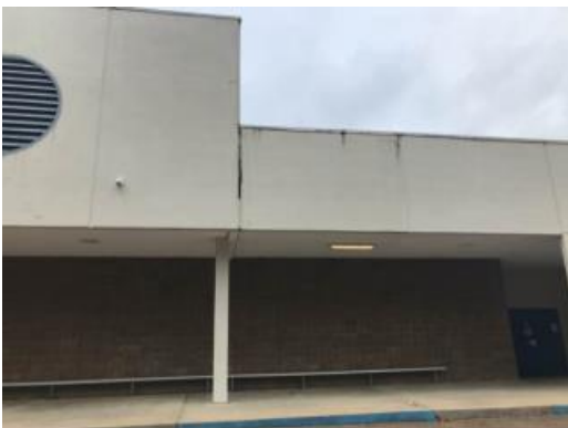
Precast panel joint damage
