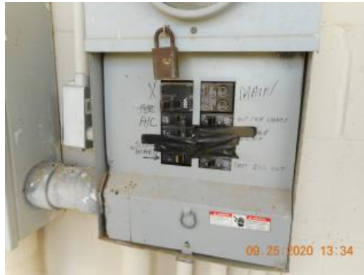
Panelboard with tape covering breaker switches
