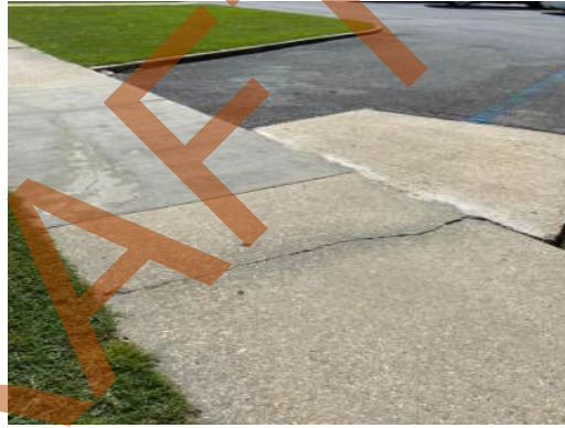
Cracked sidewalk at main entry
