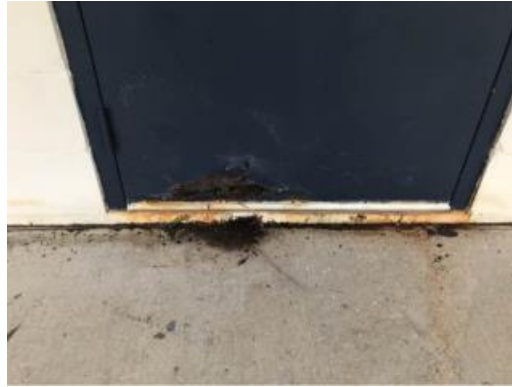
Rusted exterior door
