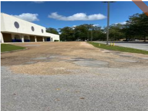
Failing asphalt south of building
