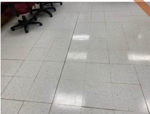
VCT separating at seams
