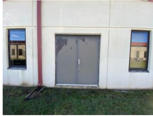
Worn exterior doors
