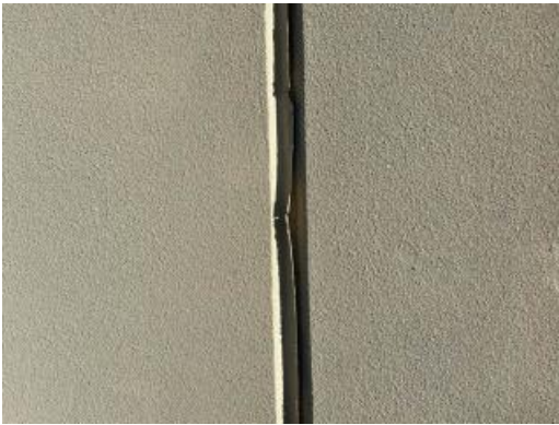
Concrete panel joint needs recaulking
