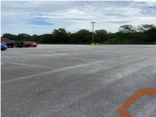
Faded striping, typical throughout parking lot
