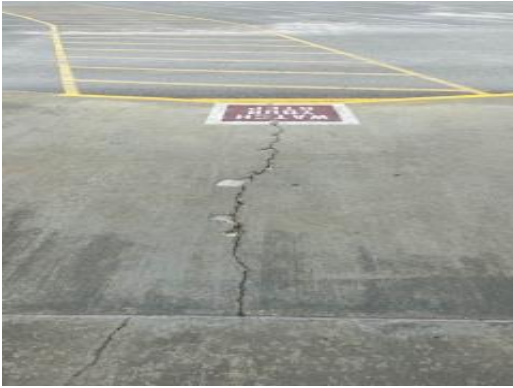
Cracked sidewalk east of main entry
