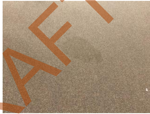
Water damaged carpet
