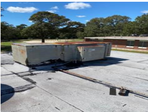
Abandoned make up air unit
