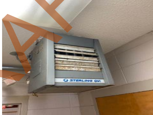
Unit heater in boys bathroom
