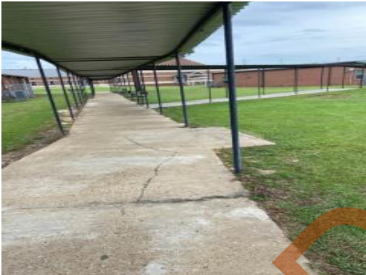
Cracked sidewalk north of Bldg K
