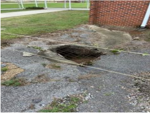
Site drainage issue south of Bldg B
