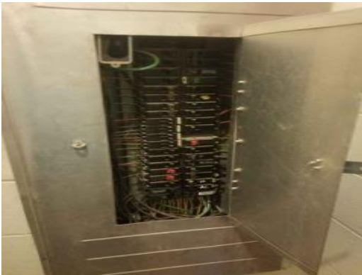
Panel missing deadfront
