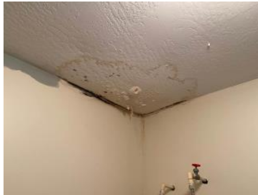
Water damaged ceiling
