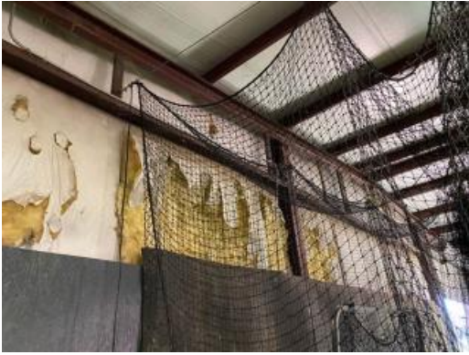
Multiple holes and tears in insulation
