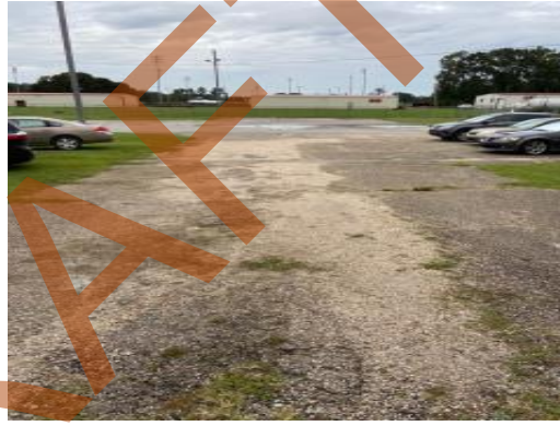
Asphalt failure north of cafeteria wing
