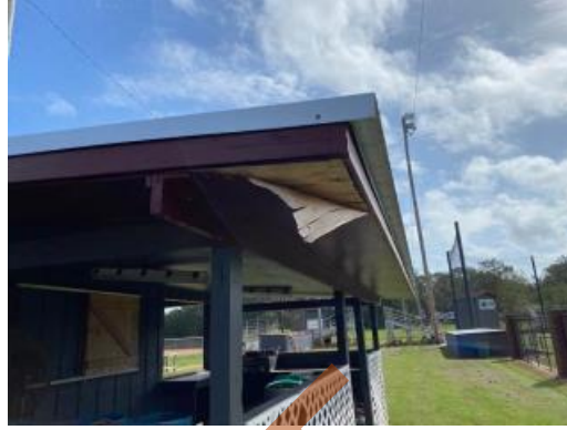
Deteriorated plywood soffit
