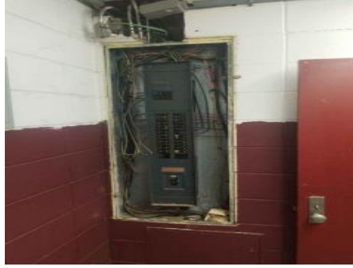
Deadfront and panel cover missing
