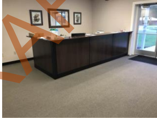
Lobby counter height not ADA compliant
