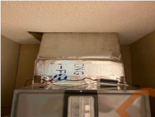
Ductwork to the air handler
