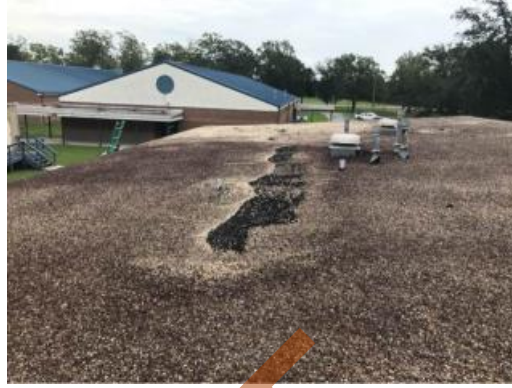
Ponding on roof
