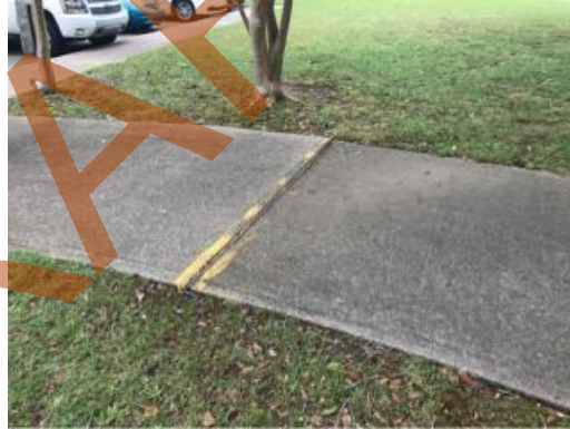
Sidewalk trip hazard
