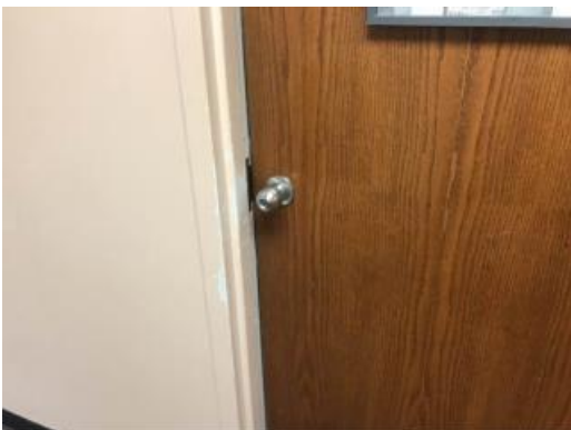
Doors lacking ADA hardware throughout
