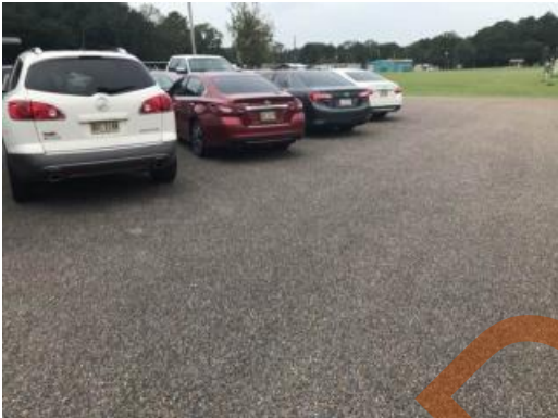
Faded parking lot striping
