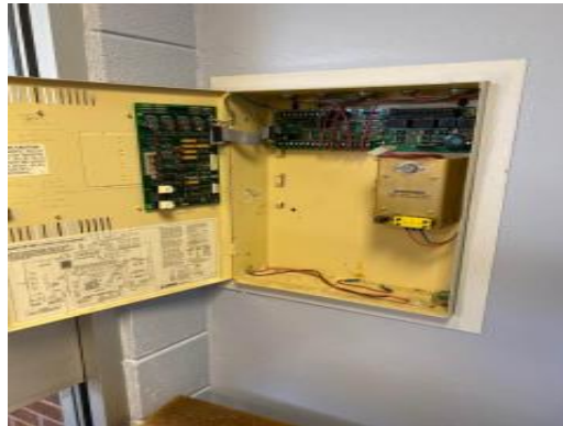
Non-functional fire panel
