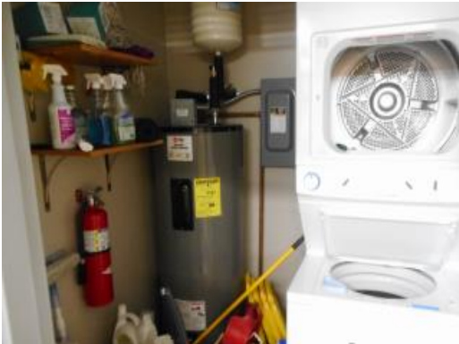
Fab Lab utility closet with water heater
